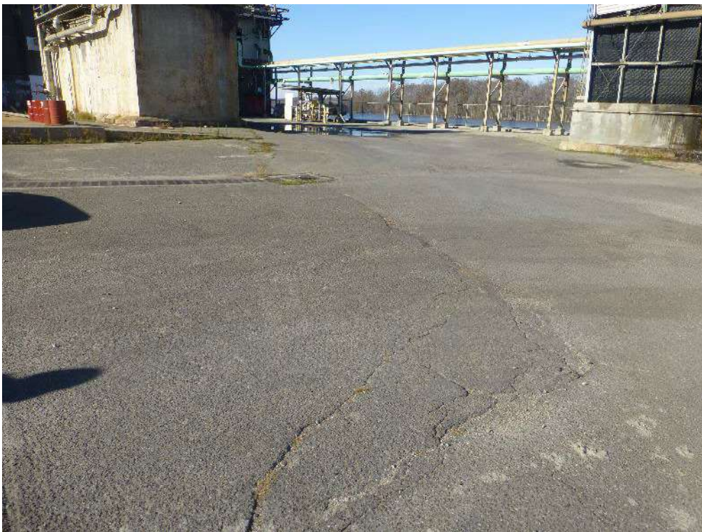
Asphalt cap at the former chlorine plant (OU-3); the seam in the asphalt shows the location of the subsurface barrier wall
