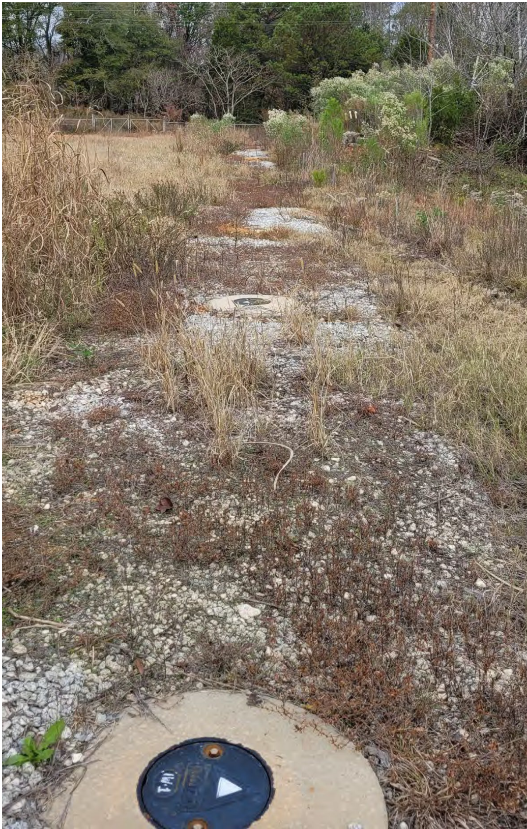
Site Photograph N4 - Infiltration Area 2 Injection Wells
