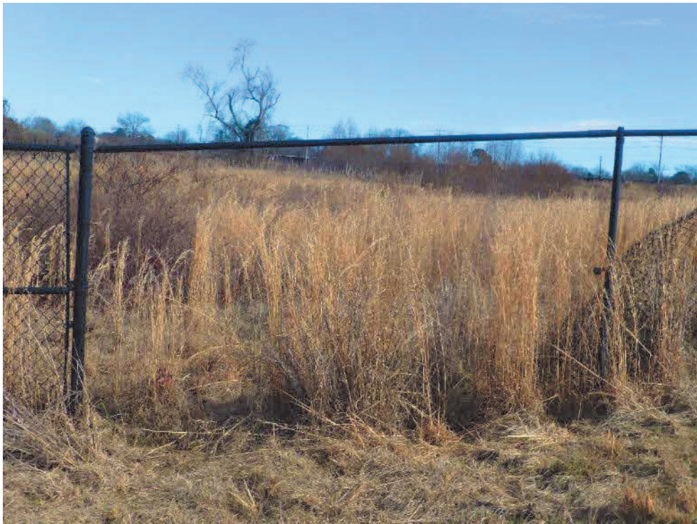
Hole in cap perimeter fence near MW-3
