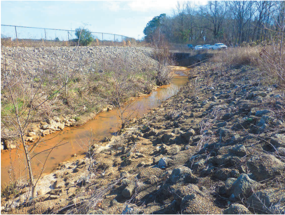
Stabilized creek banks along Hughes Creek, looking toward the culvert and sheet piling wall
