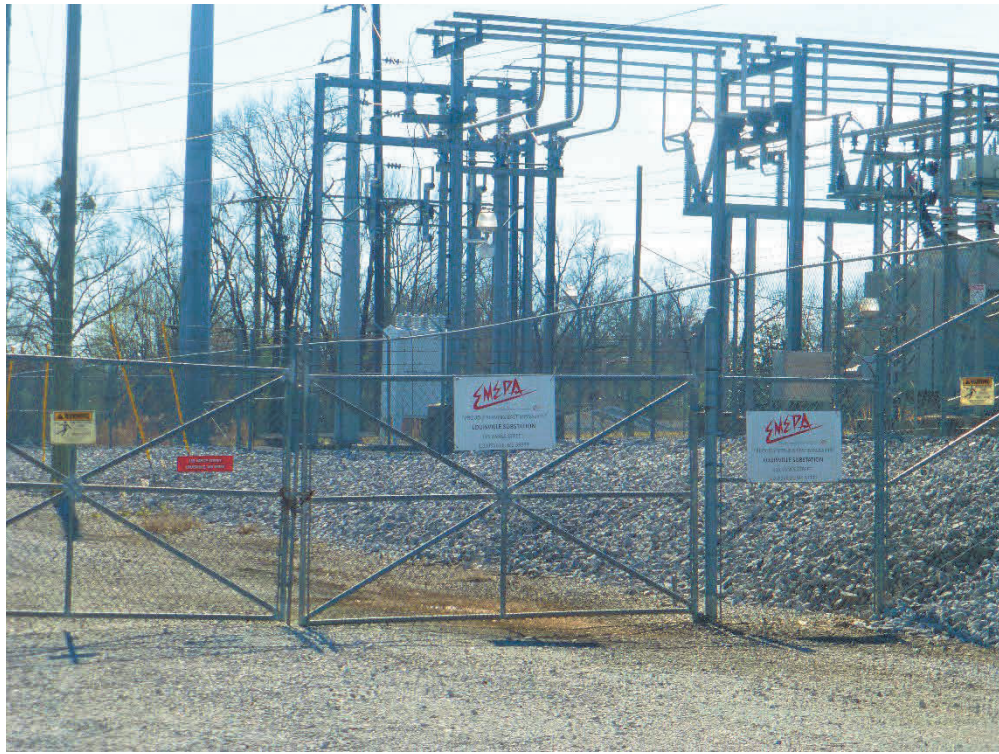
Electrical substation on north end of the Site
