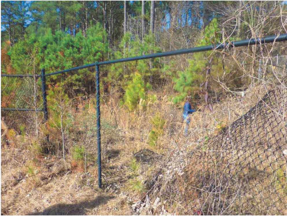
Hole in the cap perimeter fence near nearby church
