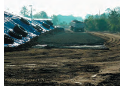
View looking east at the south haul road from Thomas street as a dump truck leaves the site after dumping a load of crusher run road base material. 4/19/2007
