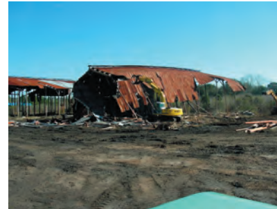
Looking northeast as the Kobelco SK 210 excavator, with grappler jaws, finishes pushing down pole barn #7. 2/22/2007
