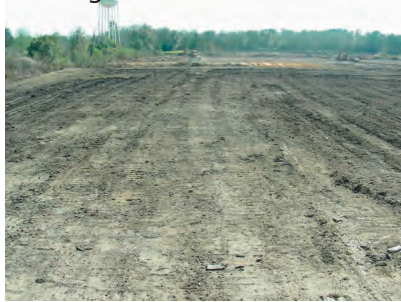
Looking south from the edge of the drip pad zone at the clean up of the pole barn area. 2/27/2007
