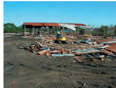
General view looking north, showing pole barns #6 and #7 debris and pole barn #8 remaining to be demolished. 2/22/2007
