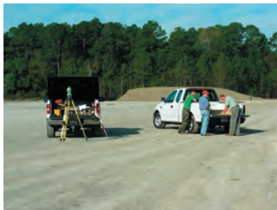
View of Camilla's consulting engineering surveyors setting up to begin the lay out for the proposed soccer fields. 3/21/2007
