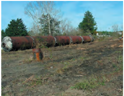
View looking North of the 8' x 120' vessel and site as the Cat D5 Dozer removes vegetation in preparation to move the wood-preserving retort or vessel to the remedial site that is located just across Thomas Street to the West. 1/11/2007
