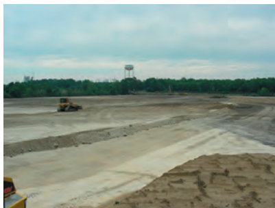
Looking southeast, as the Cat D-6 dozer builds and grades the western soccer field. 4/18/2007
