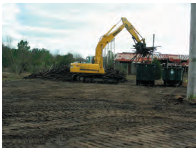
Looking South as the Kobelco SK210 Excavator with the grappler continuing with the loading of the roll-off dumpsters. 1/13/2007
