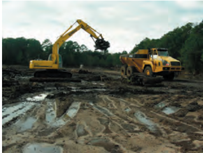
View of the Kobelco SK210 Track Excavator loading the Moxy Articulating Dump Truck with poles from the drip track area. 1/6/2007
