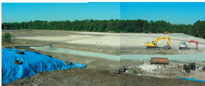
General view looking west at the progress of the construction of the soccer field and parking area. 4/21/2007
