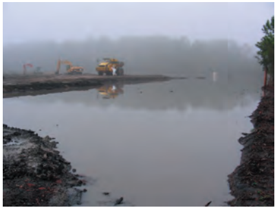
General view, looking East, shows the flooded drip track excavated area after a rain. Link Belt Mini-Excavator and Cat 320 Excavator, excavating relief channels for drainage. 1/6/2007
