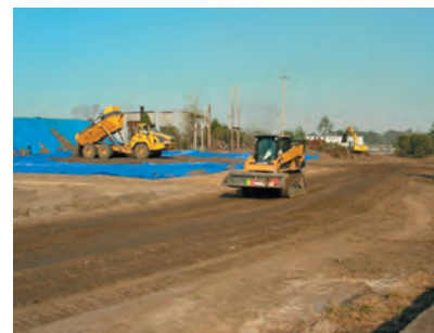
Looking east at the Moxy articulating dump truck as it dumps a load of contaminated material in the second stockpile. The Kobelco SK210 excavator, with grappler jaws, continues with the stockpiling of debris. 3/5/2007
