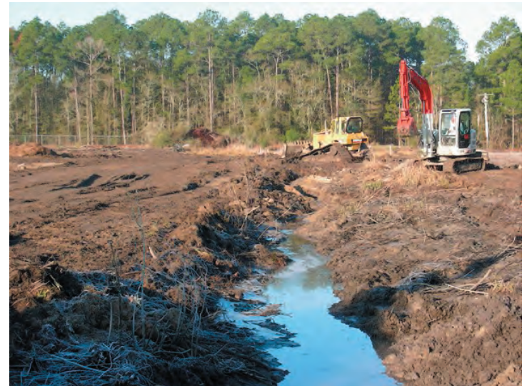
Looking west along the ditch alignment that is located next to the drip track zone, as the Cat D-6 bulldozer begins to fill it in with its berm material. (Courtesy of EPA, 2/27/07)
