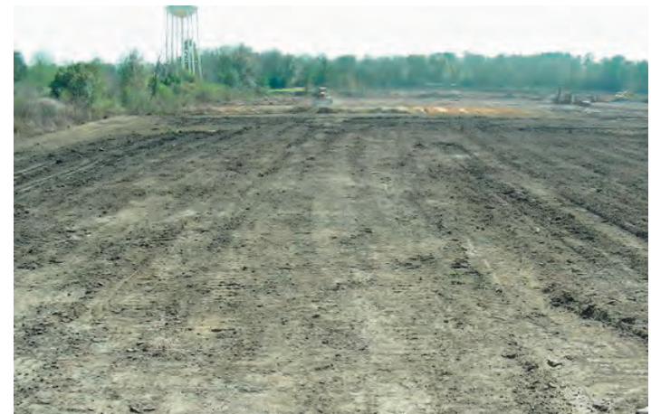
Looking south from the edge of the drip track zone at the clean up of the pole barn area. (Courtesy of EPA, 2/27/07)
