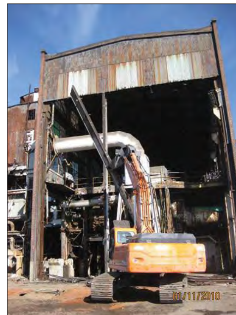
EPA successfully removed all permanent buildings on site to protect human safety and facilitate the productive reuse of the property.
