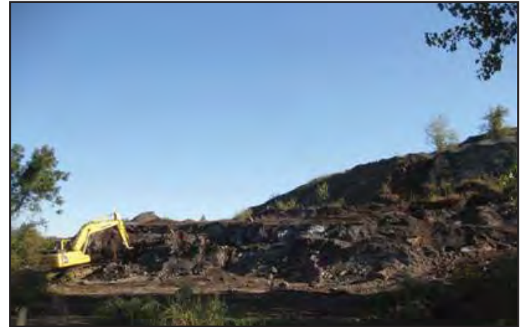
EPA conducted a metal recovery pilot and identified a cost-effective and feasible method for removing the slag piles over a two to three year period.
