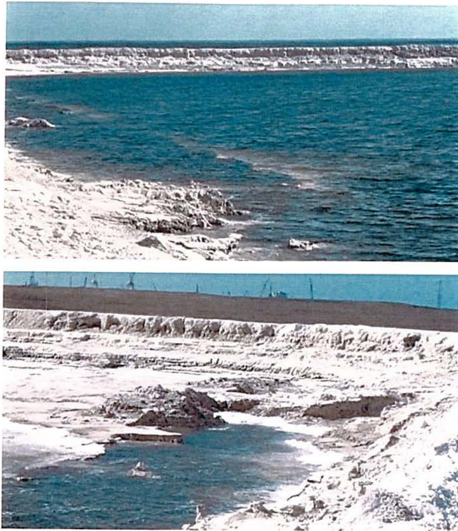
Figure 6. Photos of Pond 3 at the EGS showing wave cut steepening and erosion of the containment dike taken on October 5, 2017. Top: Looking east at northeast dike wall; Bottom: Looking southwest at southwest dike wall.
