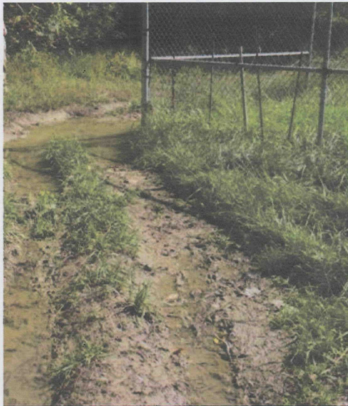
Ponding water and raised/missing fence on the eastern portion of the Site.
