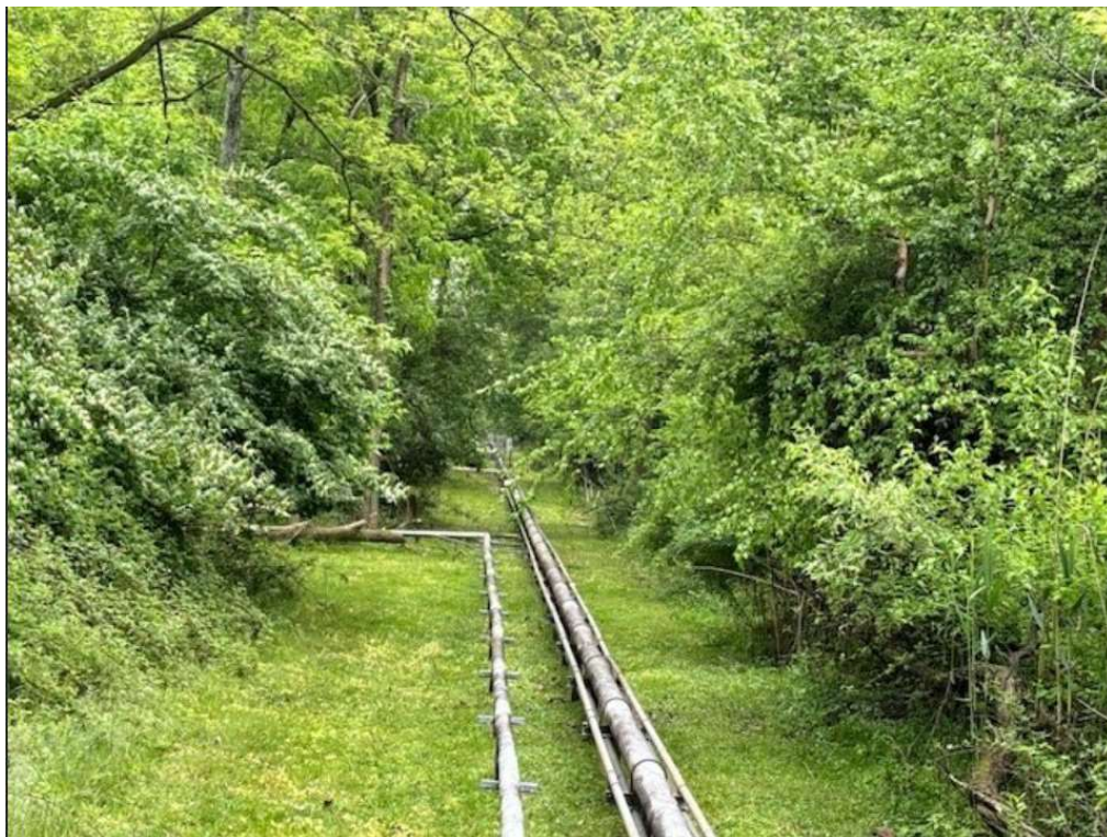
Recovery well water transfer pipes
