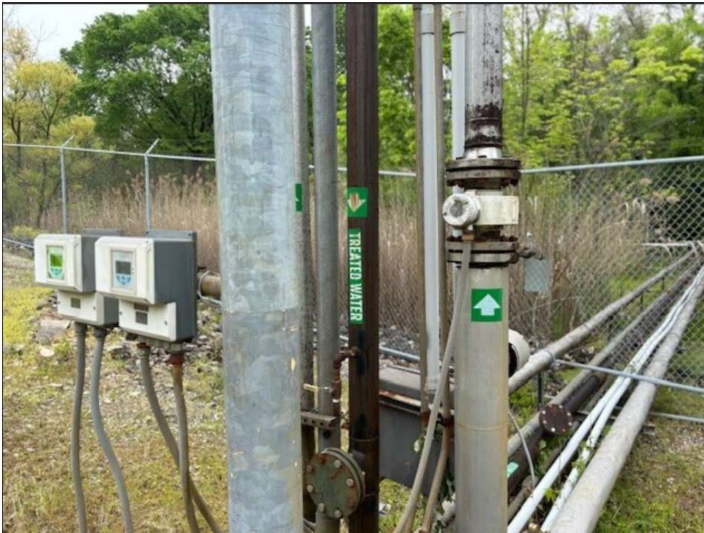
Effluent flow meter and totalizer
