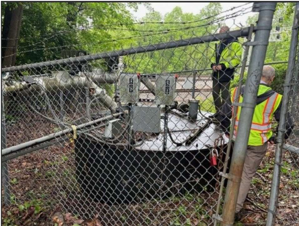
Seep water collection tank
