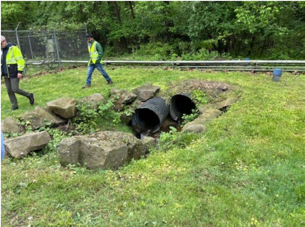
Storm water control
