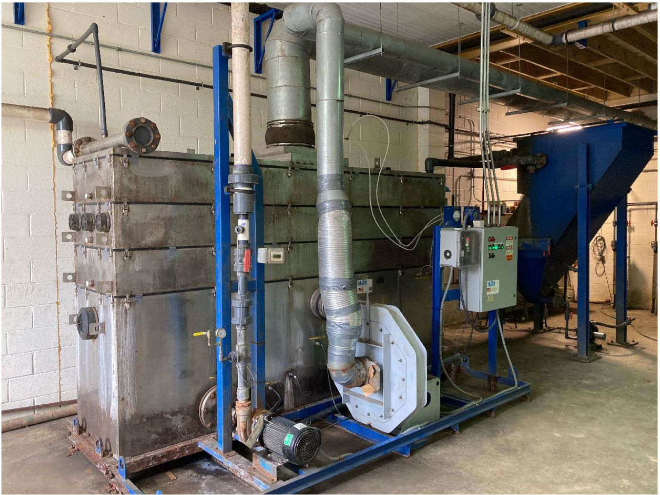
Water treatment plant air stripper
