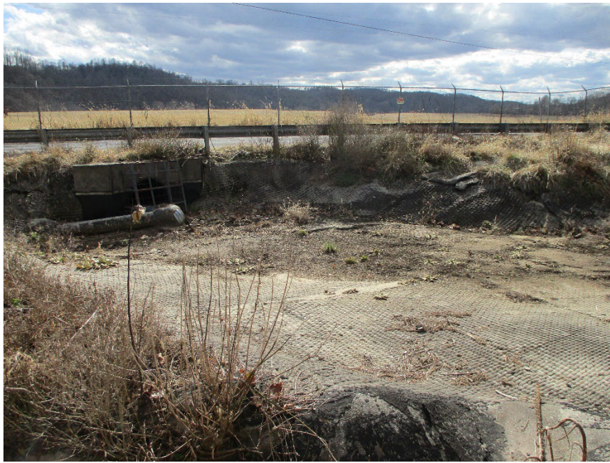
Swale 1 Interceptor System, grout blanket damaged and geomembrane exposed (facing south)
