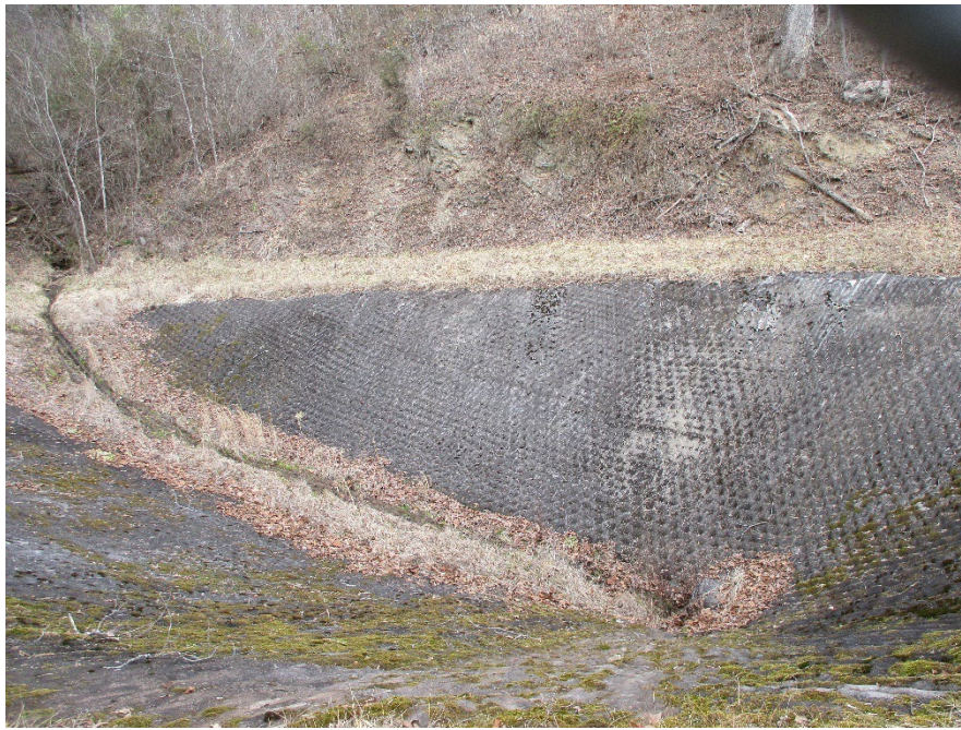
Swale 3 Interceptor System
