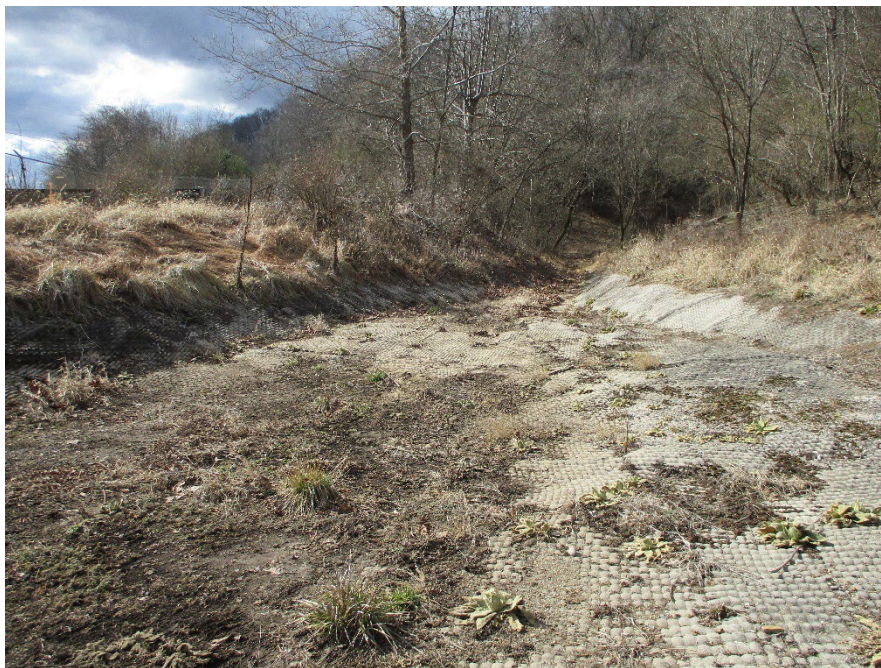
Swale 1 Interceptor System, grout blanket damaged and geomembrane exposed (facing northwest)
