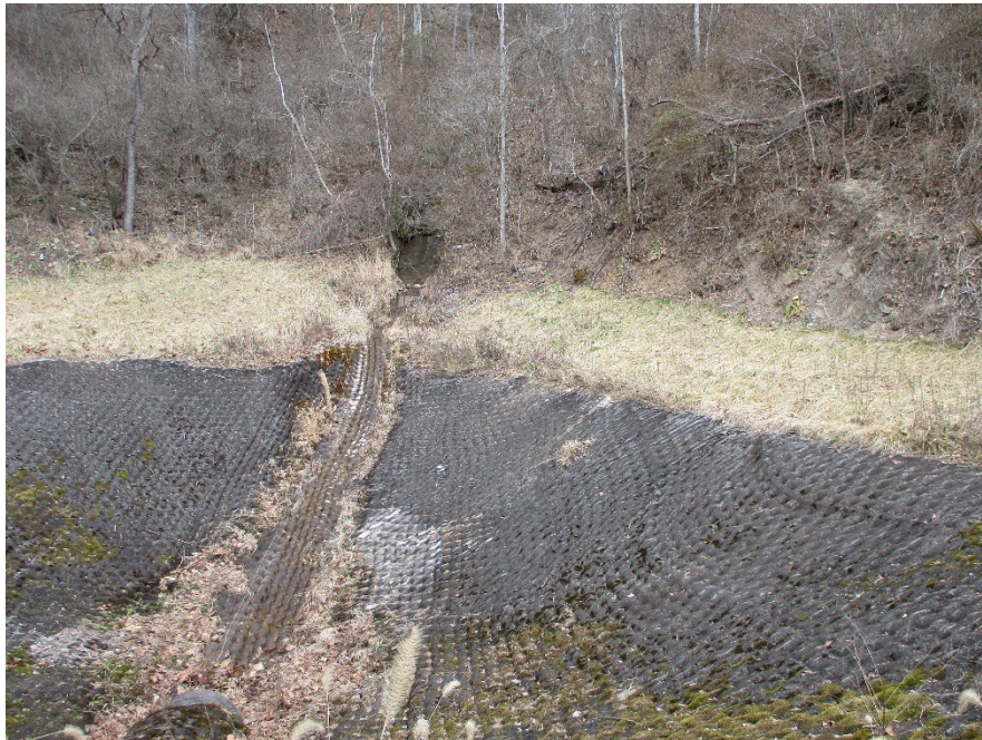
Swale 2 Interceptor System
