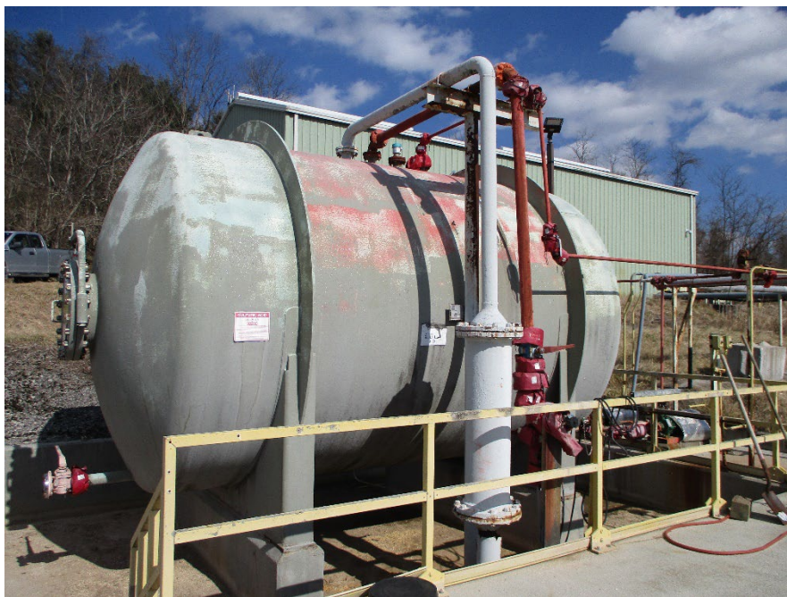
Acid feed tank
