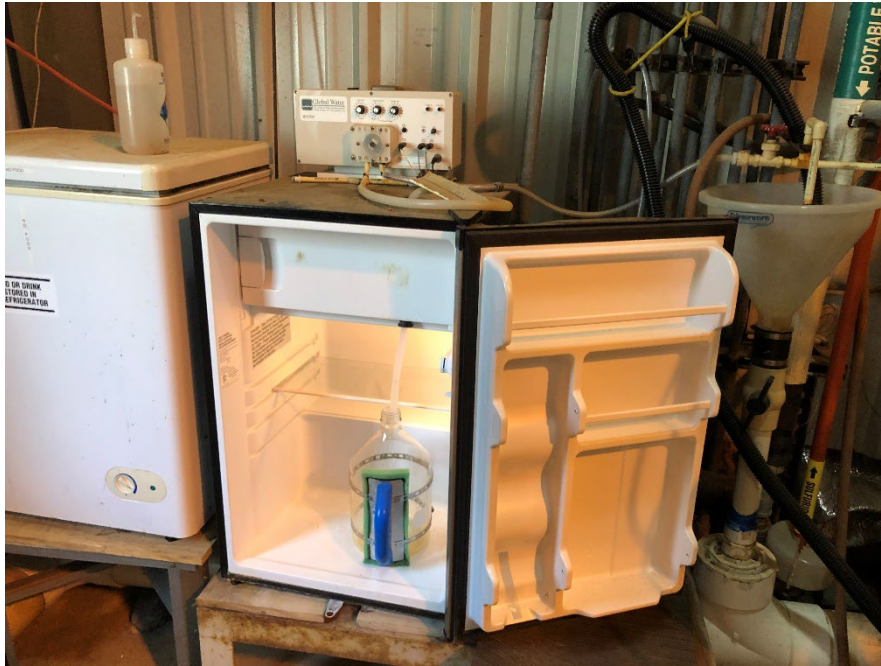
Daily composite water sample system inside SSTP
