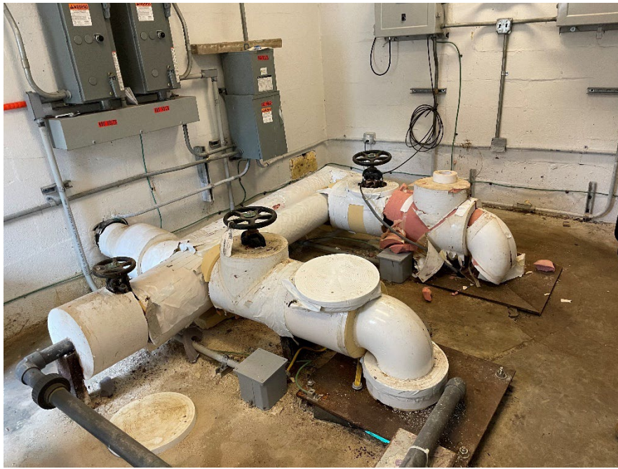
Inside Pond 6 pumping station
