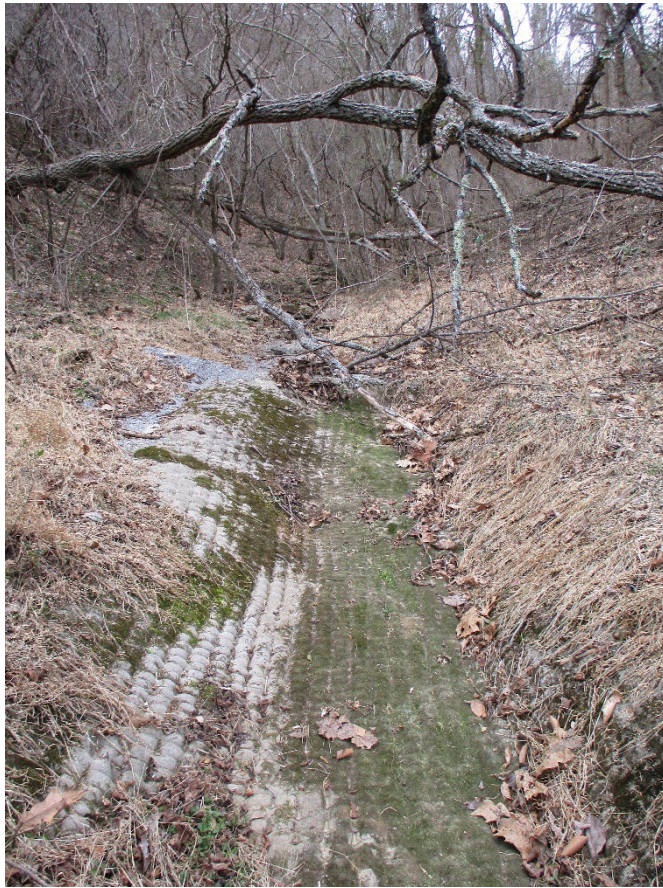
Swale 1 Interceptor System, grout blanket damaged and geomembrane exposed (facing north)
