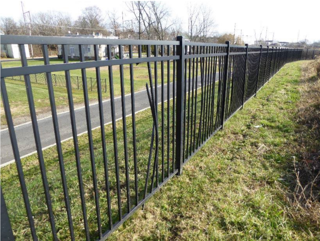
Damaged fence at Park Parcel
