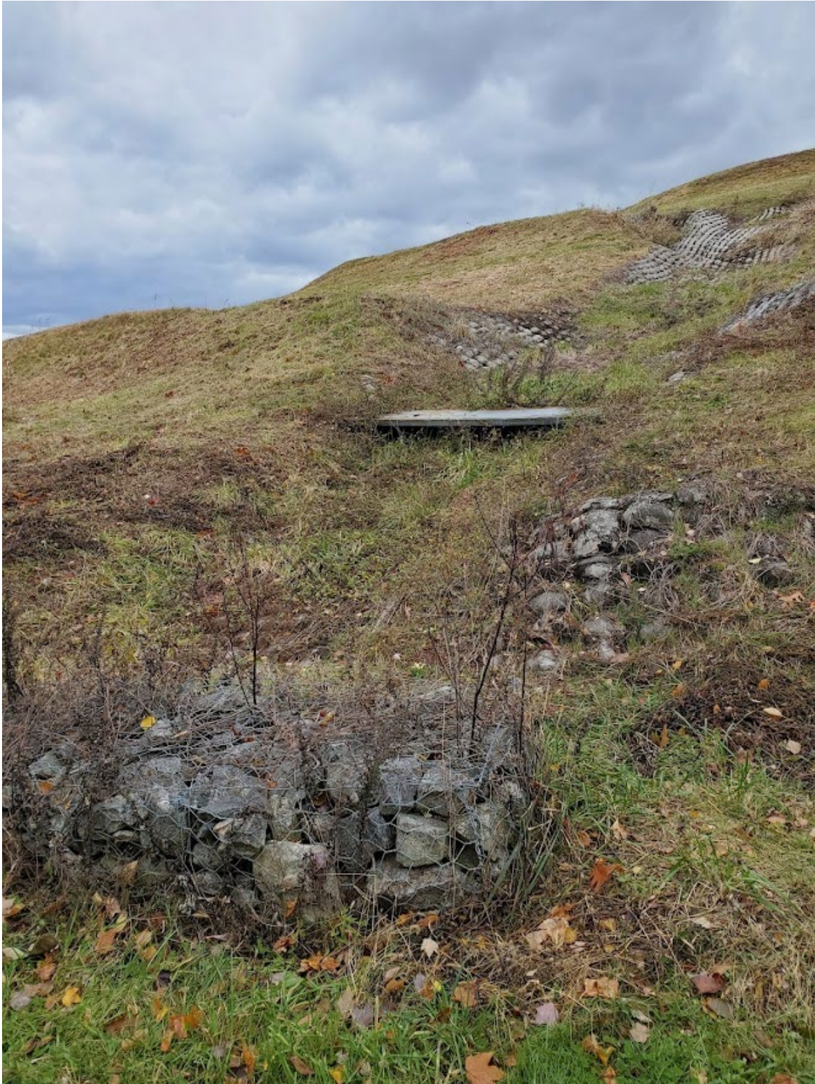
Grout bag on East side covered in vegetation
