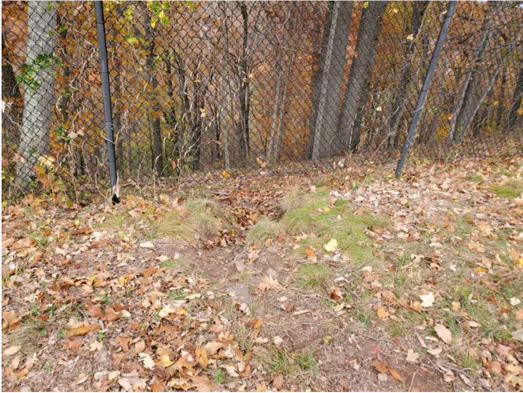
Erosion under fence on West side
