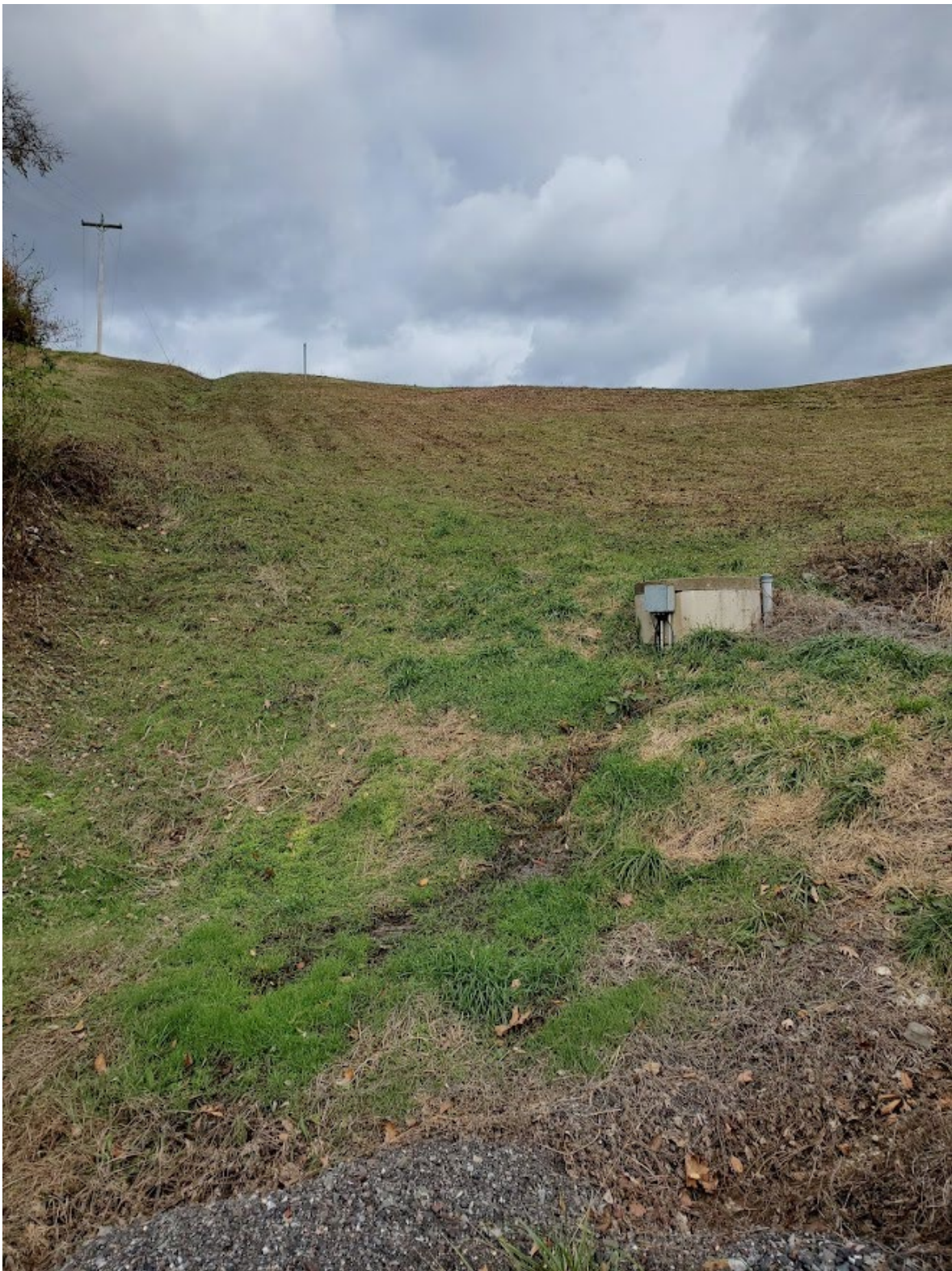
Overflow of leachate discharge from South Valley manhole
