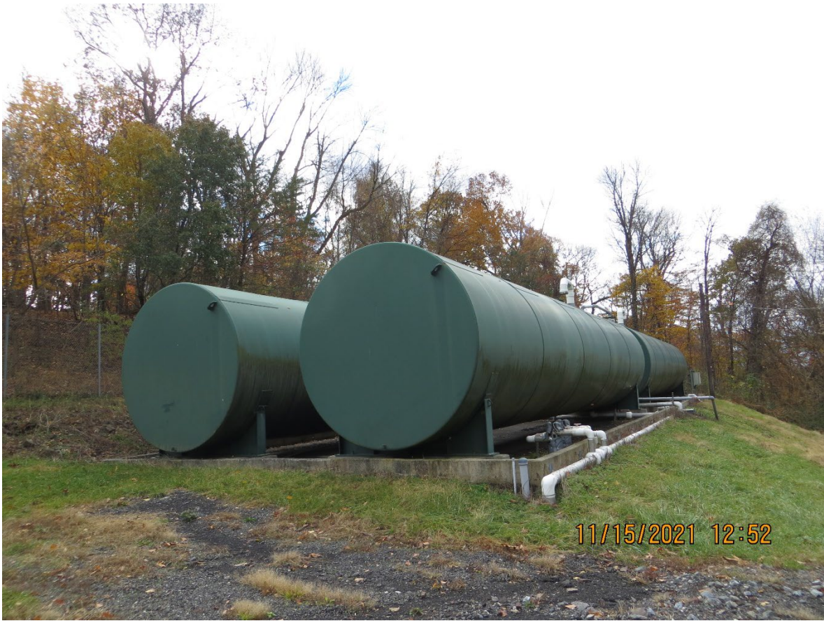
Leachate holding tanks
