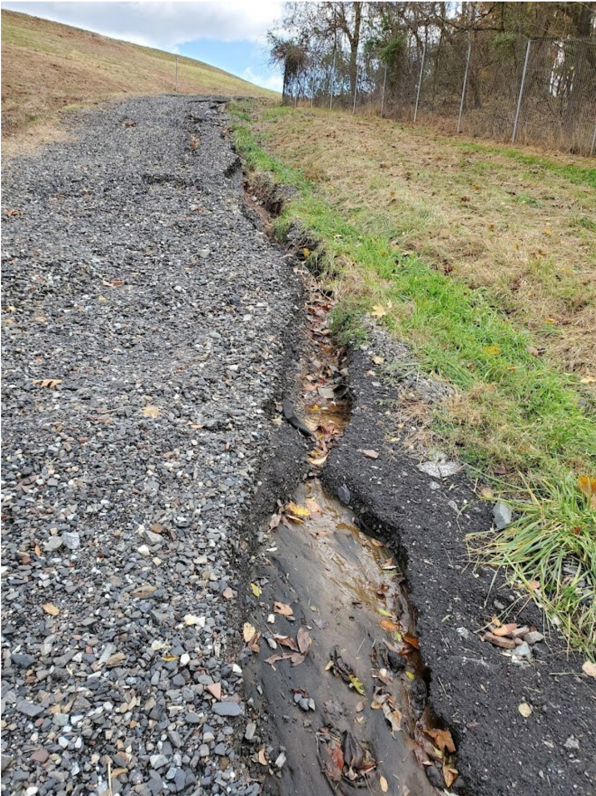
South Valley access road erosion
