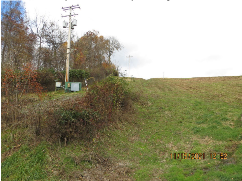
South Valley pump station off
