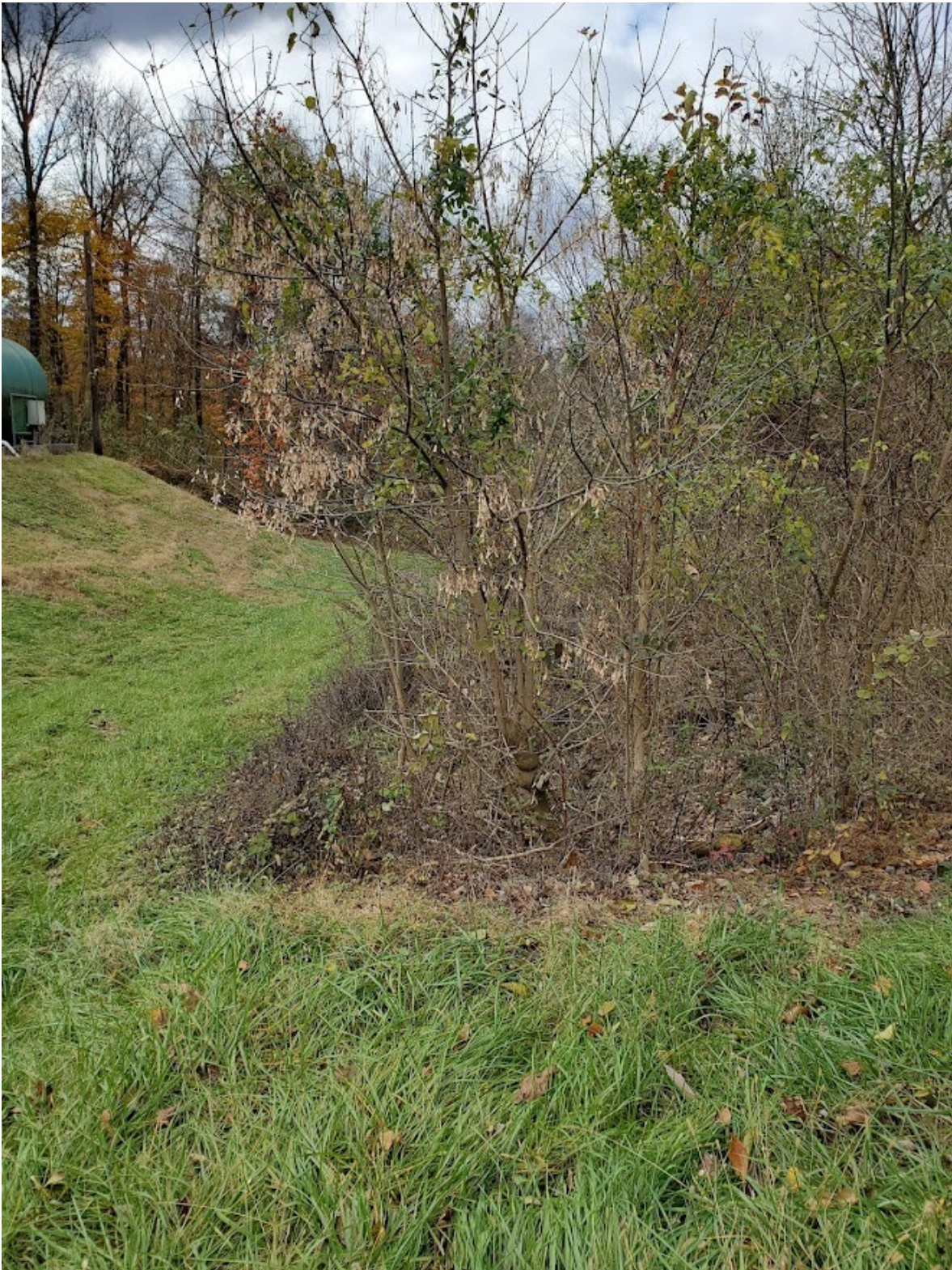
Overgrown drainage basin in South Valley
