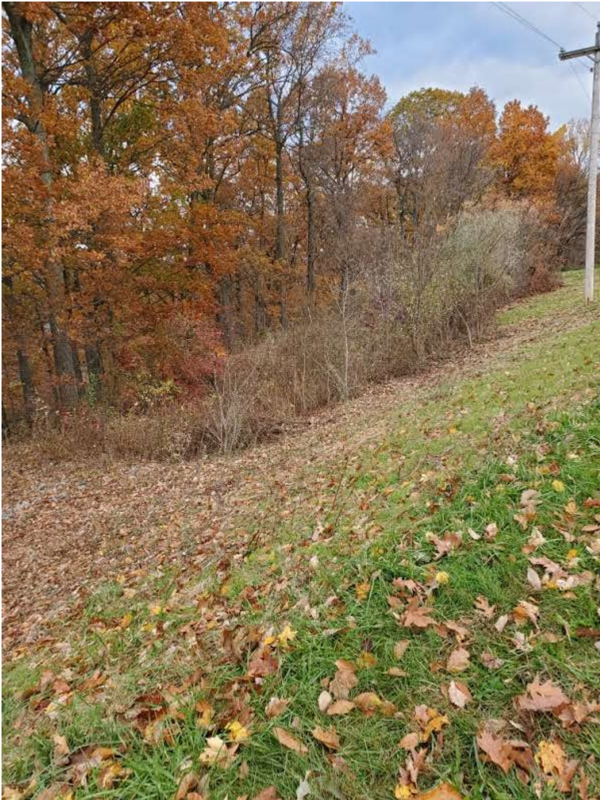
Overgrown drainage basin on West side
