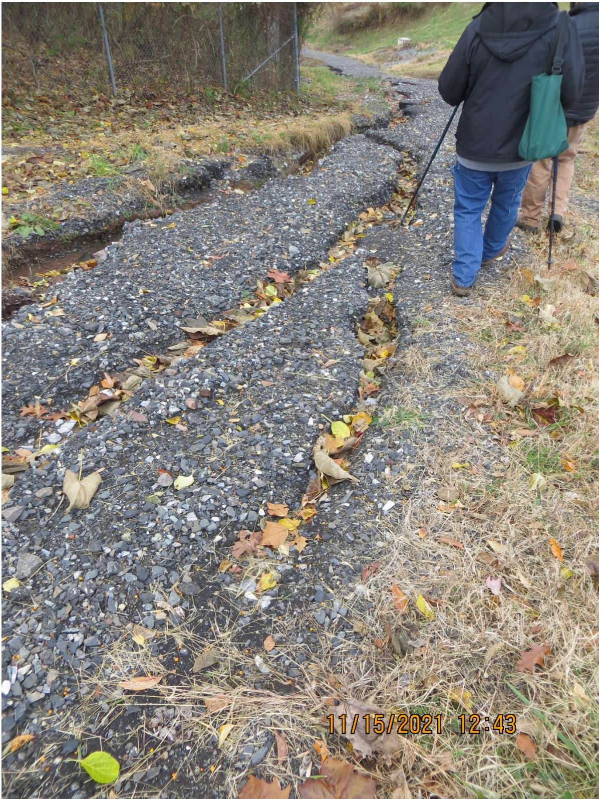
South Valley access road erosion
