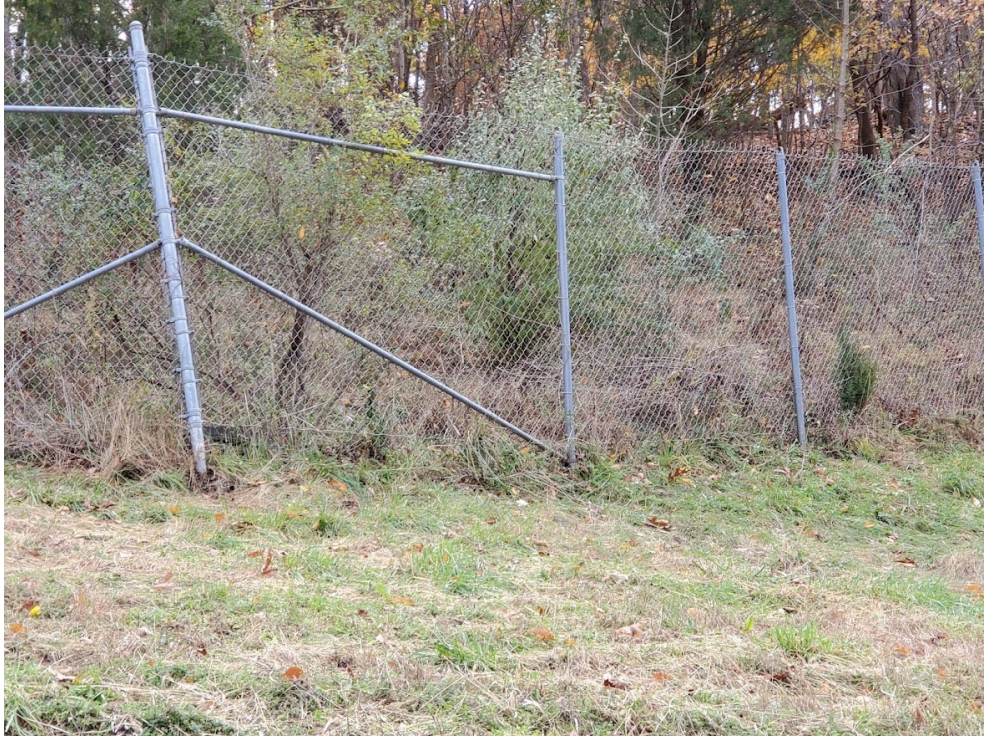
Gap between South Valley fence and ground
