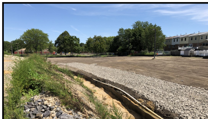
Repairs made to fill in the damage caused to Eastwick City Park near Apollo Place. (Photo from August 24, 2020)
