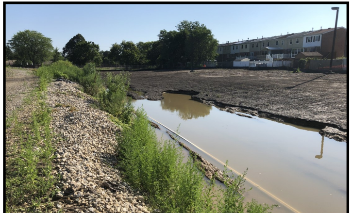
Close-up showing erosion of clean soil from Eastwick City Park near Apollo Place after flooding. (Photo from August 5, 2020)
