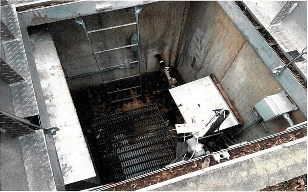
Picture 6. Pumping well (PW-08).
