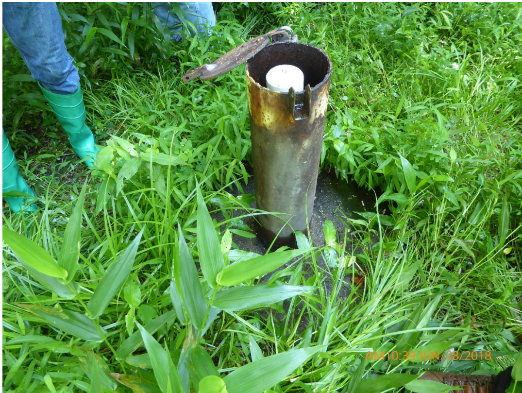
Monitoring well MW 18-1 with unsecured well stickup lid
