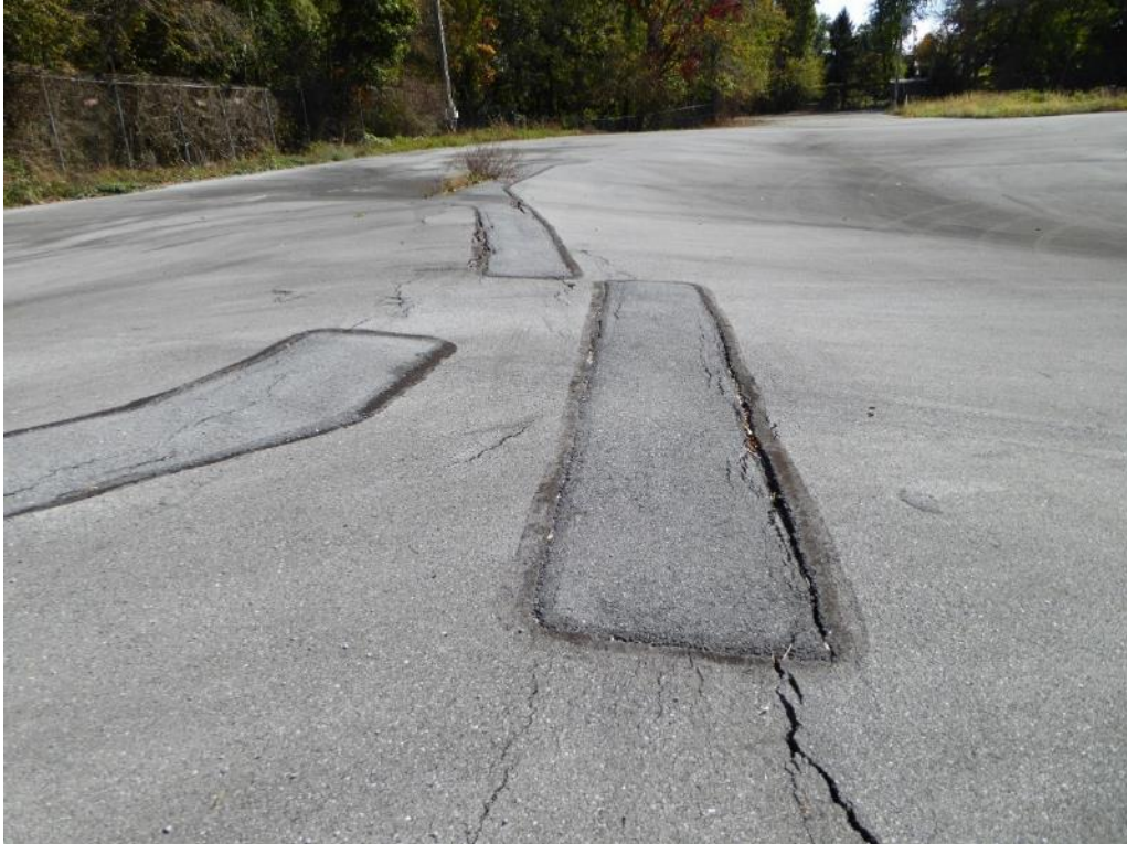
Cracks in previously repaired area of asphalt cap.
