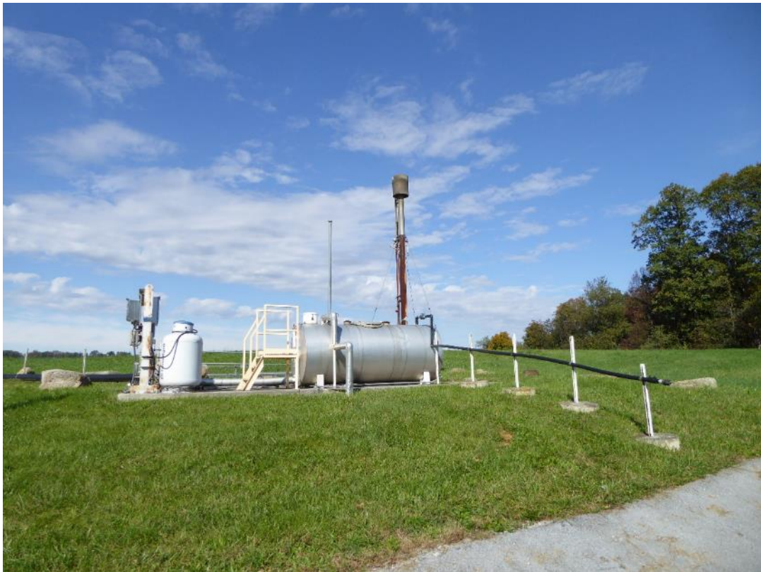
Landfill gas flare (in operation).
