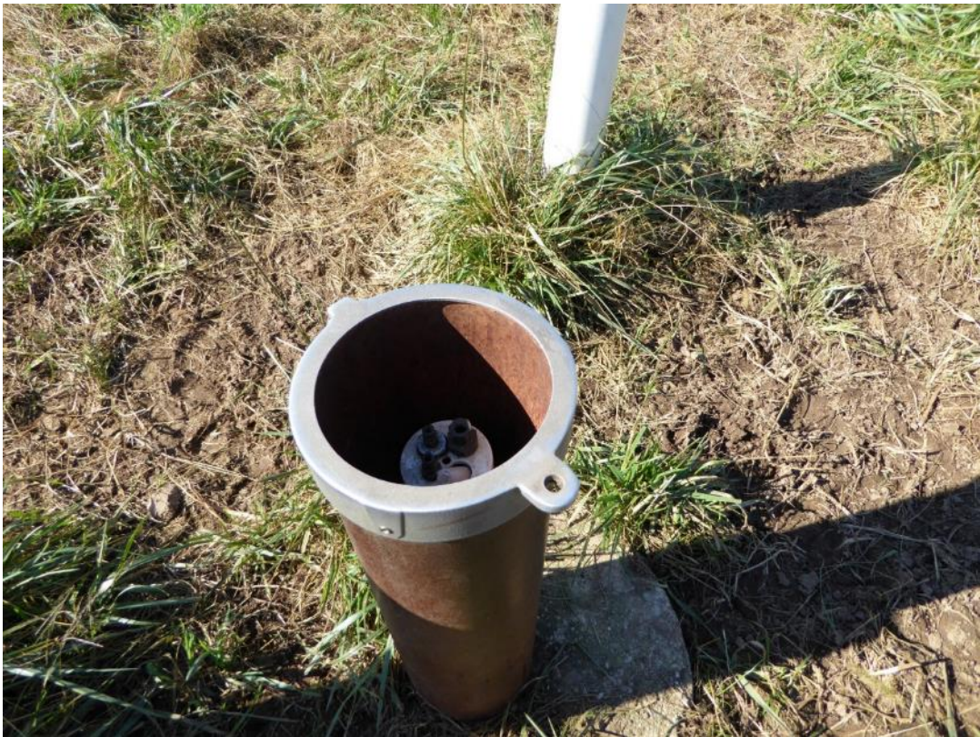
Monitoring well (missing cap).
