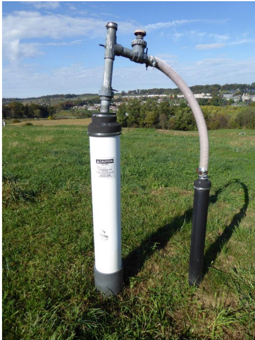
Landfill gas collection well.
