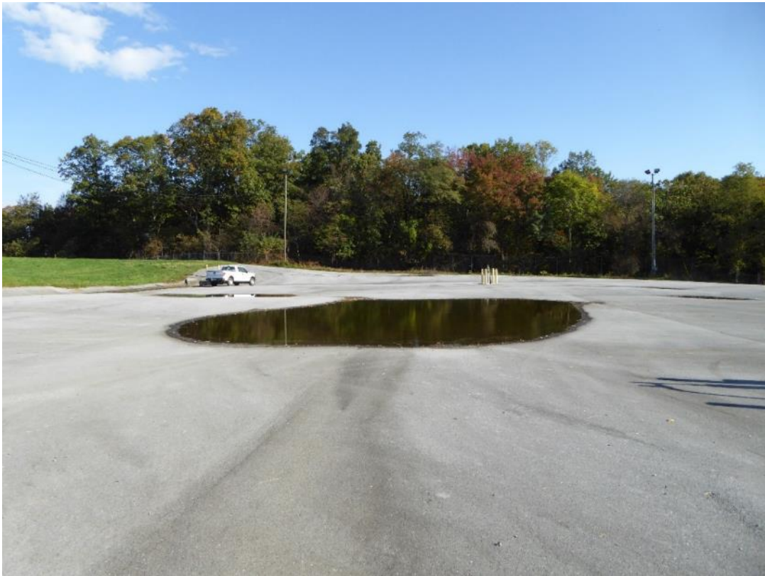
Ponded water on asphalt cap.
