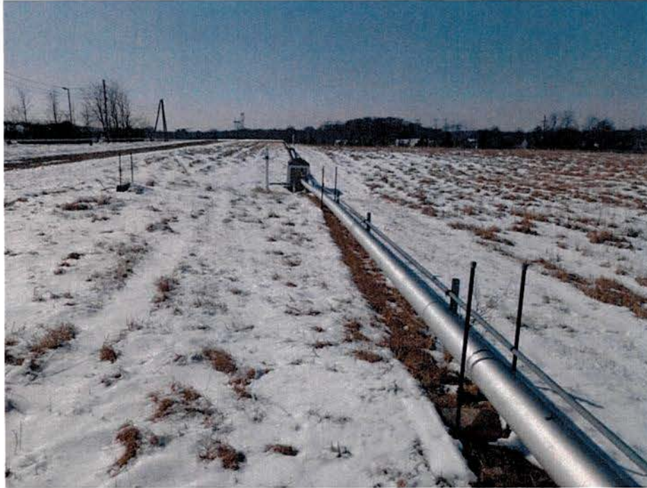
This main line transports landfill gas from the perimeter of the landfill to the landfill gas stack at the center of the landfill.
