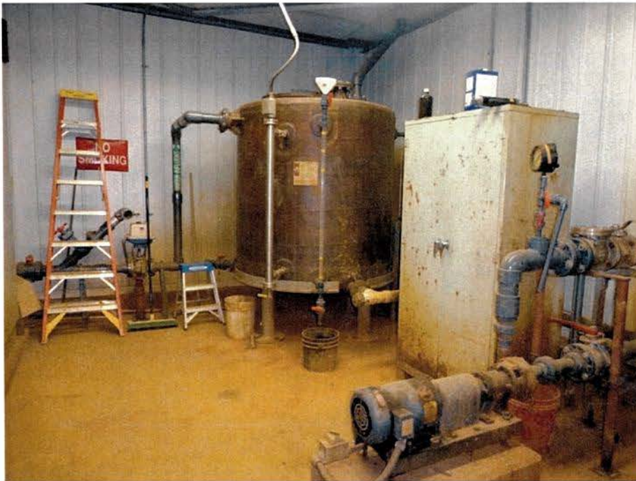
Equalization tank inside of the inactive pump house.
