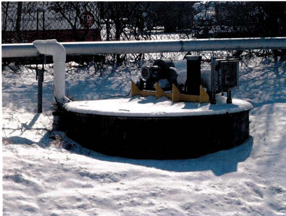
IW-8, located near the blower building, is one of the several interceptor wells around the Site that are no longer in operation.
