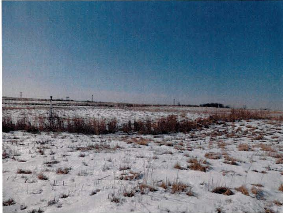
Another area of cap settlement was observed along the landfill's southeastern edge.
