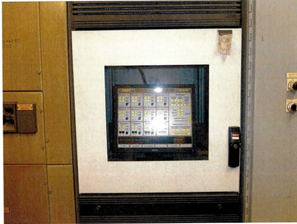
This programmable logic controller monitors the landfill GMCS and sends system status reports to the PRP office daily.
