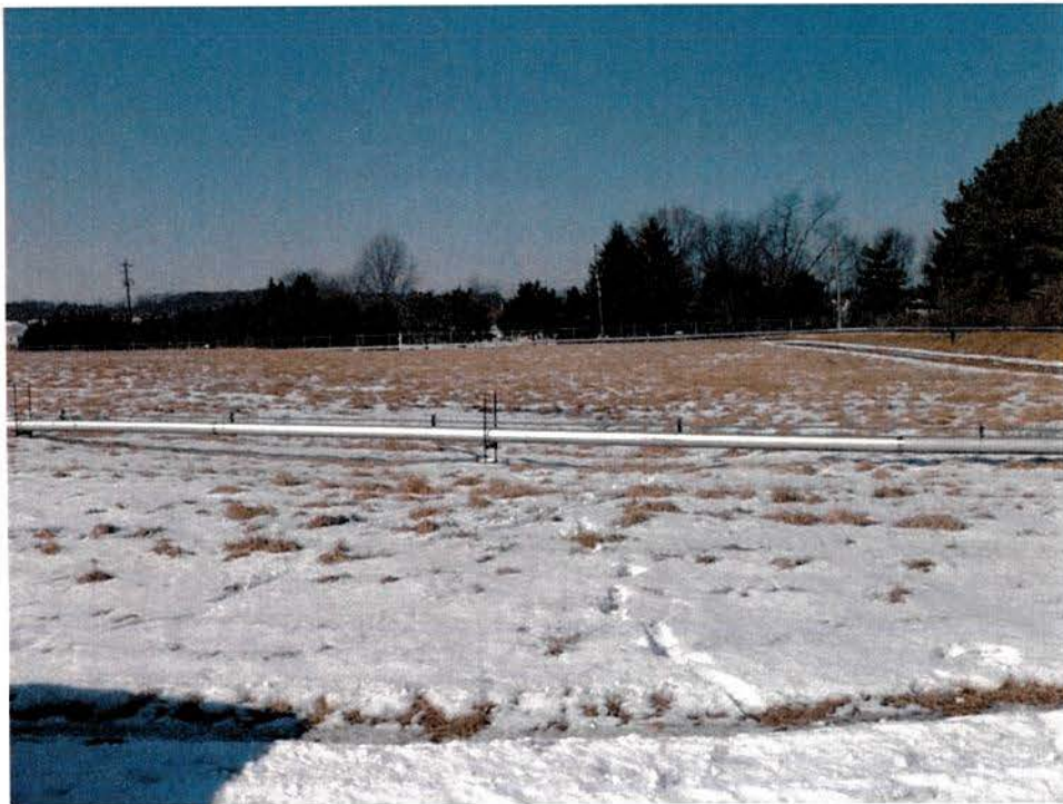
An area of subsidence is located immediately west of the blower building, at the far northern end of the landfill.
