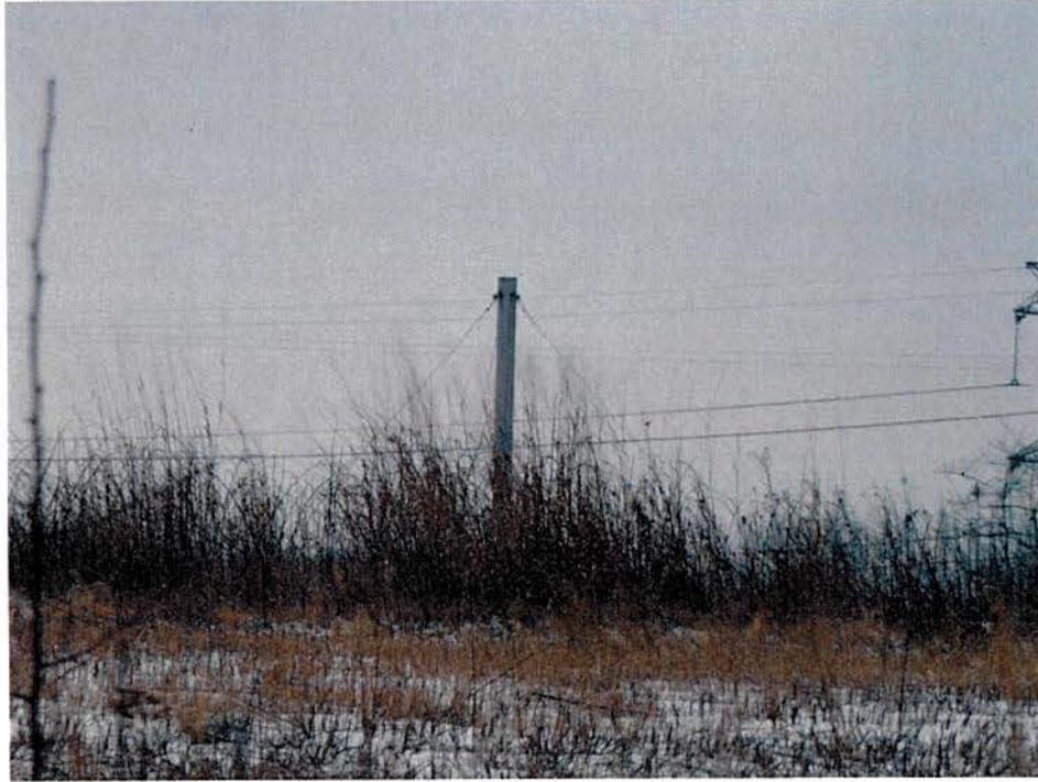
Landfill gas pulled in from the perimeter of the landfill is pumped through piping to this central stack.
