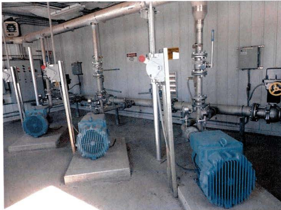
Interior of the blower building.
