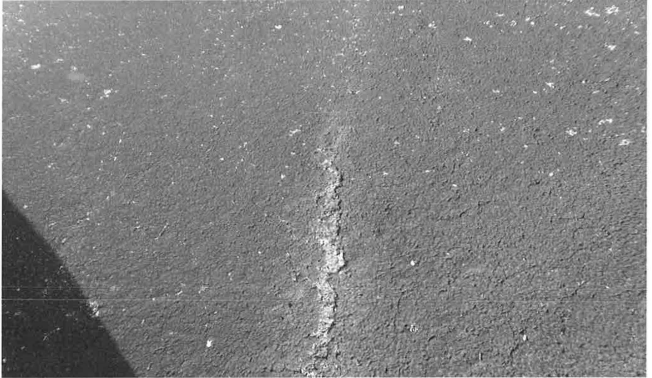
Hellertown Manufacturing Co. Superfund Site - Fourth Five-Year Review Minor Surface Cracking in Paved Former Lagoons Area
