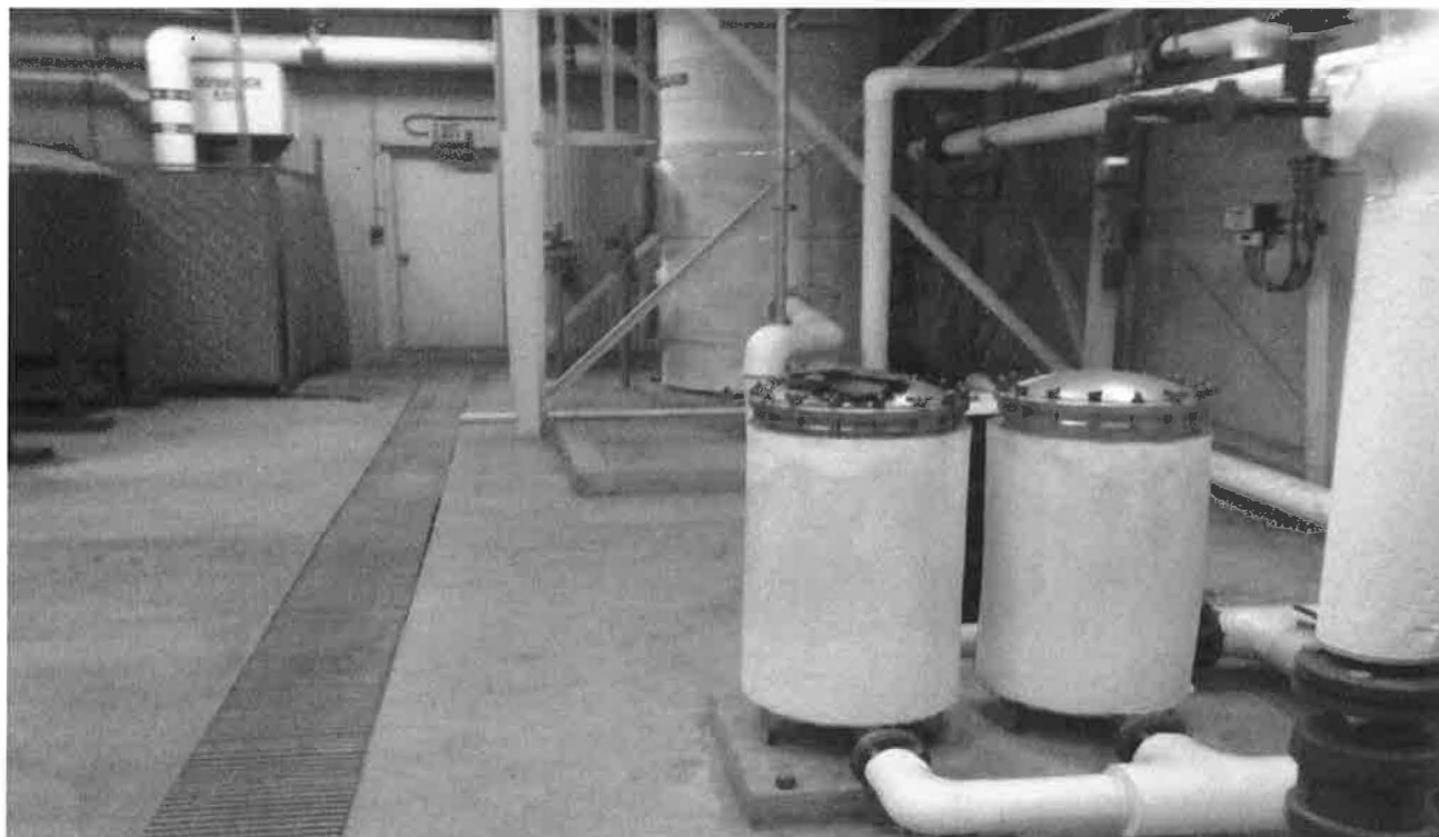
Hellertown Manufacturing Co. Superfund Site - Fourth Five-Year Review Groundwater Treatment Plant – Cartridge Filters and Air Stripper
