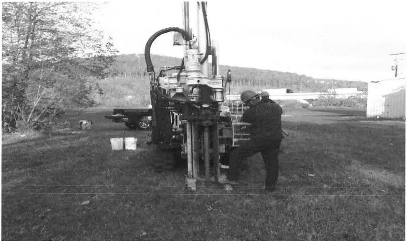
Hellertown Manufacturing Co. Superfund Site - Fourth Five-Year Review Geoprobe in Monitoring Well CSP-7 Area
