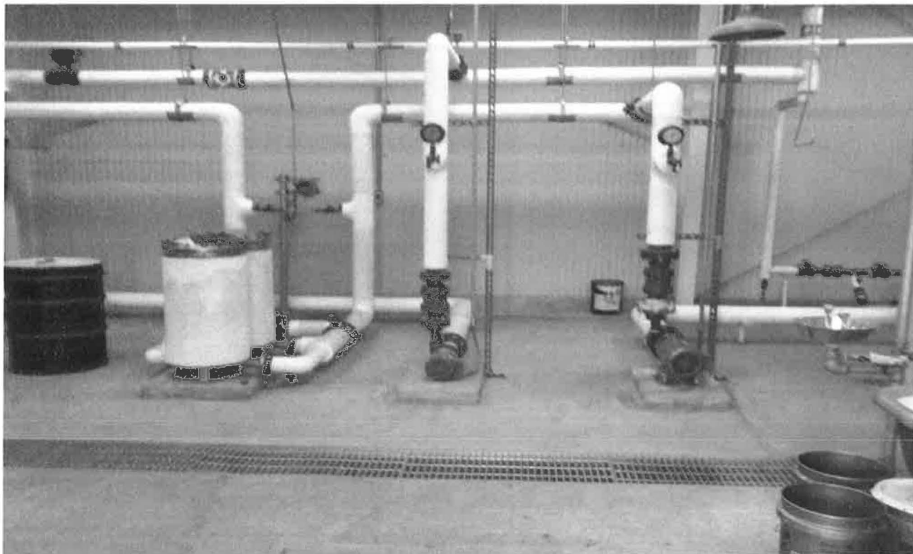
Hellertown Manufacturing Co. Superfund Site - Fourth Five-Year Review Groundwater Treatment Plant - Cartridge Filters and Process Piping
