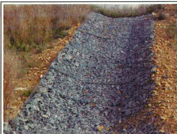
Photo 10: Viscous Basin 4, 5, and 6 (10-23-12) Latitude: 38.92959 Longitude: -78.21513 Description: Flume #3. Unstable soil
