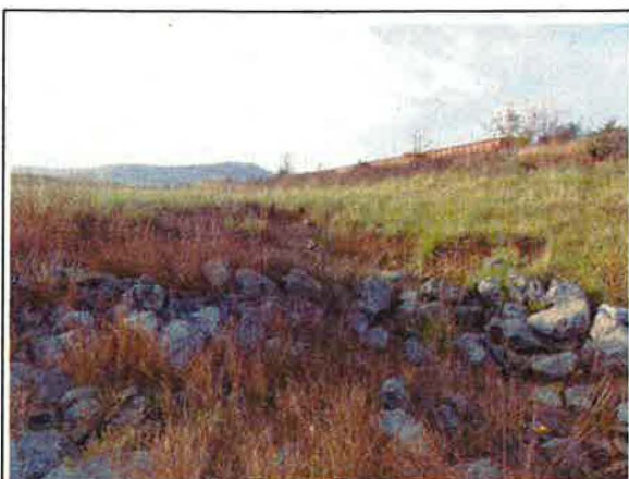
Photo 3: Storm Water Basin East (10-23-12) Latitude: 38.9221 Longitude: -78.21543 Description: Bank Erosion along Basin Inlet
