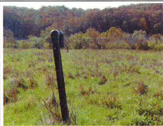
Photo 24: SB-1, Cell 4 Latitude: 38.92699 Longitude: -78.21604 Description: Gas Vent (GV25) tilting south
