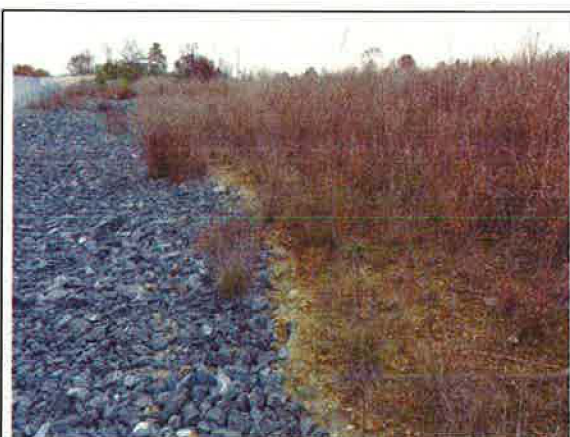
Photo 7: Viscous Basin 2 & 3 (10-23-12) Latitude: 38.92993 Longitude: -78.213 Description: Unstable soils with sparse to bare vegetation
