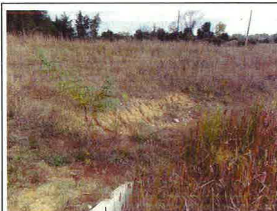
Photo 2: Storm Water Basin West (10-24-12) Latitude: 38.9221 Longitude: -78.21004 Description: Erosion Gullies North Side of Basin
