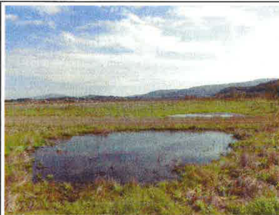
Photo 23: SB-1, Cell 3 Latitude: 38.92618 Longitude: -78.21802 Description: Surface water ponding. Settlement
