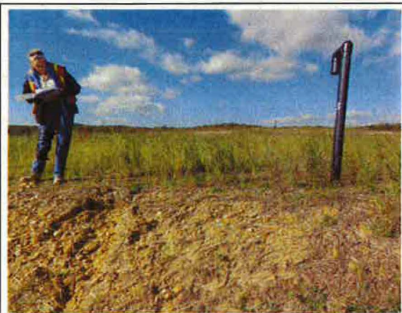
Photo 12: New Landfill (10-17-12) Latitude: not available Longitude: not available Description: Minor unstable soil & rill erosion on slopes
