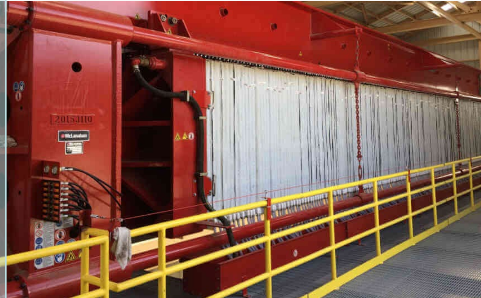
Sediment Filter Presses
