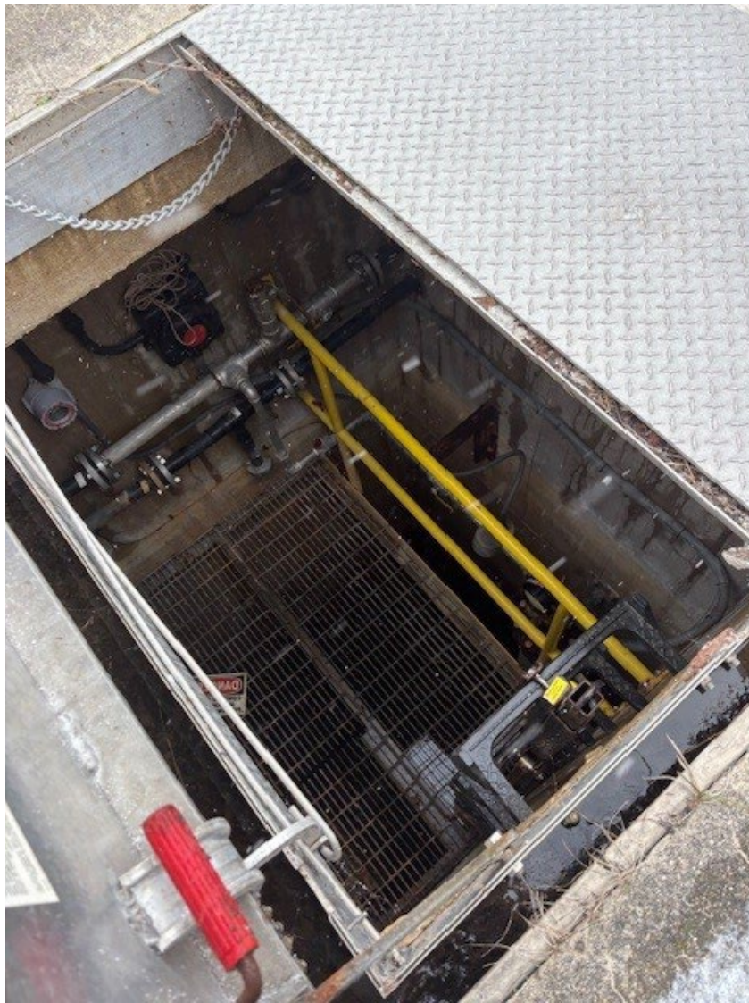
Photo 4 – Wet Well A
