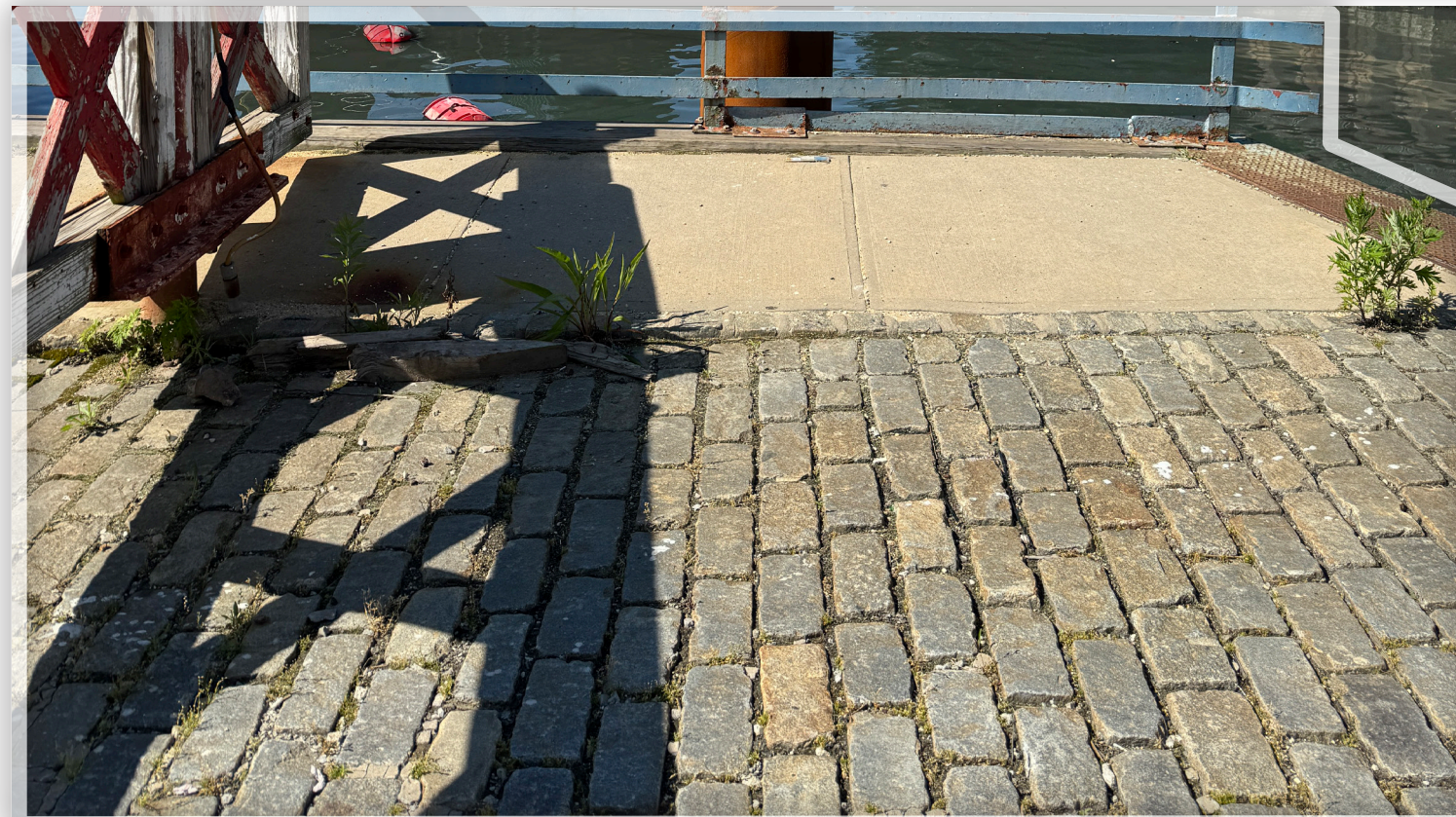
② EAST ABUTMENT VIEW LOOKING SOUTH PHOTO OF EXISTING STONE PAVERS AND SOUTH SIDEWALK
