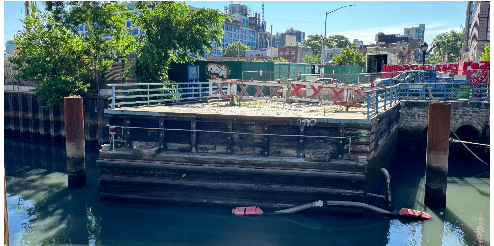
② FRONT VIEW OF EAST ABUTMENT PHOTO OF CRIBBING SETTLEMENT AT EAST ABUTMENT WEST FACE
