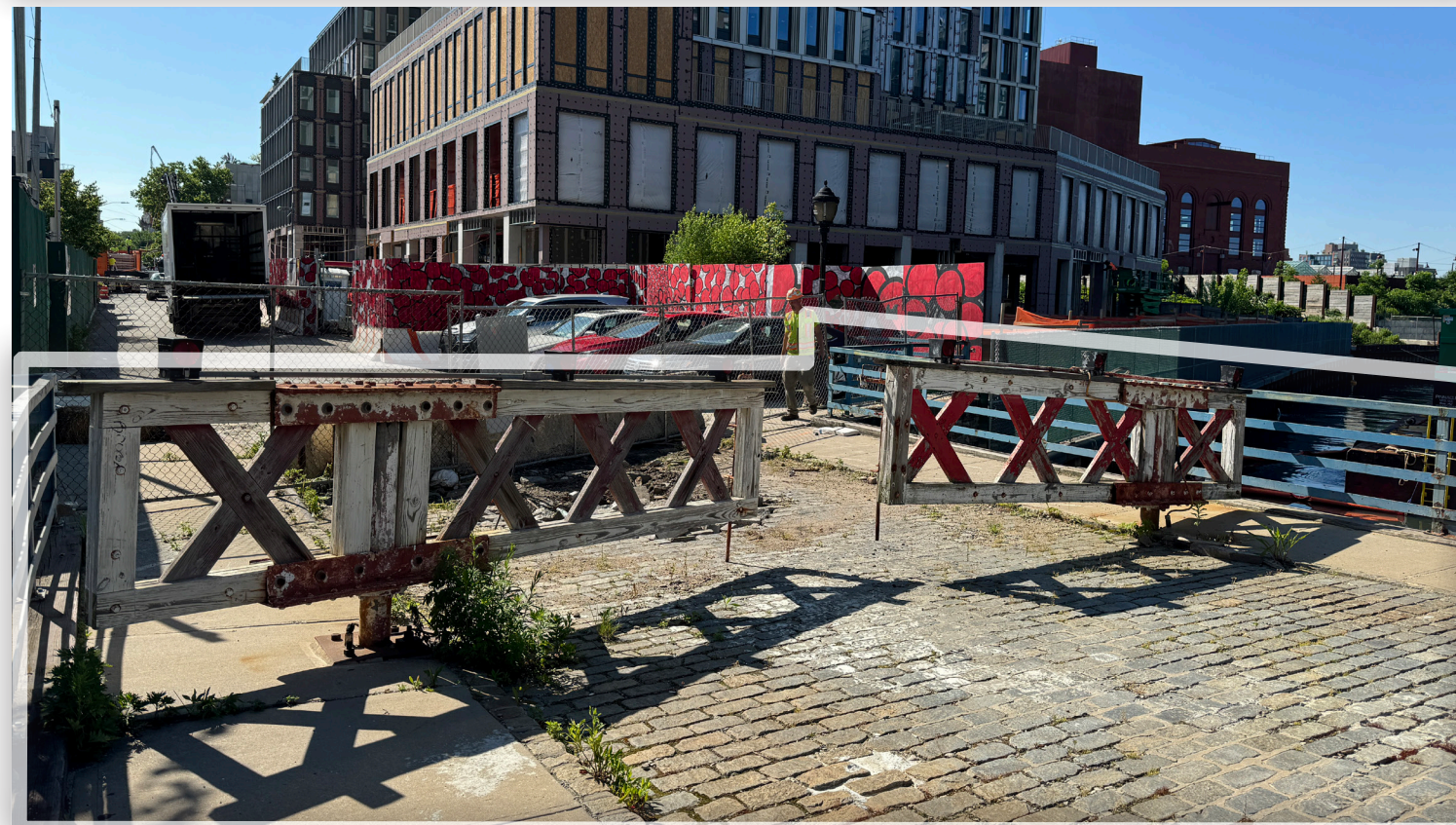
② EAST ABUTMENT VIEW LOOKING SOUTHEAST PHOTO OF EXISTING BARRIER GATE AND STONE PAVERS
