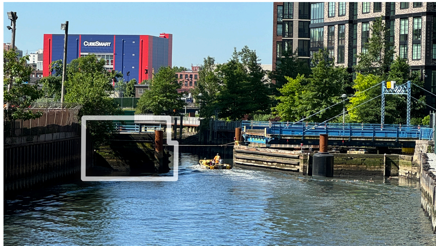
② CARROLL ST BRIDGE VIEW LOOKING SOUTH PHOTO OF BRIDGE NORTH ELEVATION FROM GOWANUS CANAL
