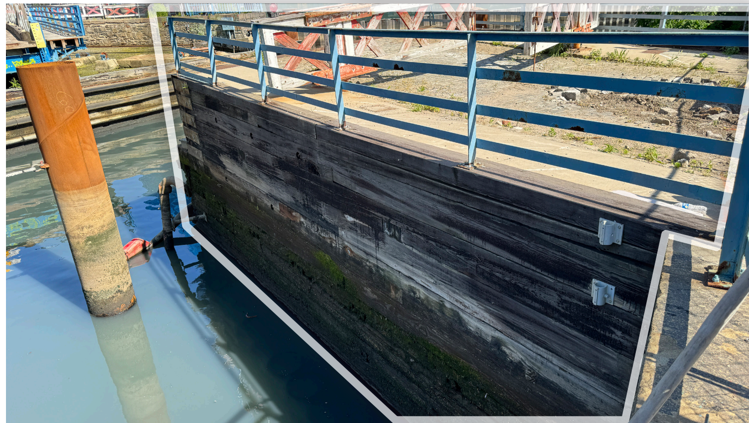
② EAST ABUTMENT VIEW LOOKING NORTHEAST PHOTO OF EXISTING WINGWALL, TIMBER CRIBBING, AND RAILING
