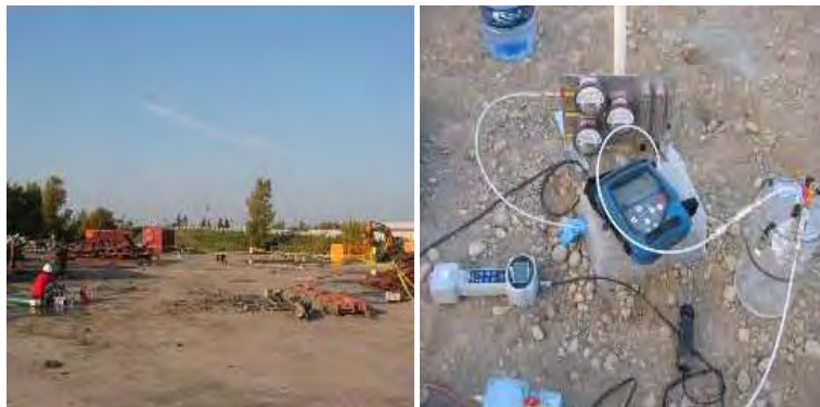
Geosyntec conducted soil gas sampling to assess the vapor intrusion potential at a Brownfield site that played a key role in constructing a safe building.
