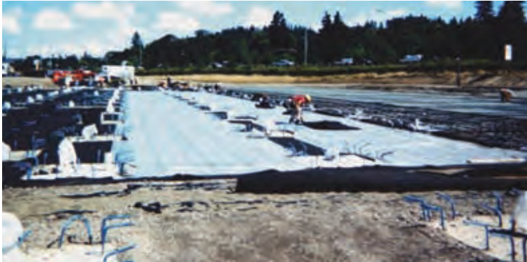
Design and installation of a vapor protection and detection system allowed productive redevelopment of the closed Rossman's Landfill as a Home Depot retail site.
