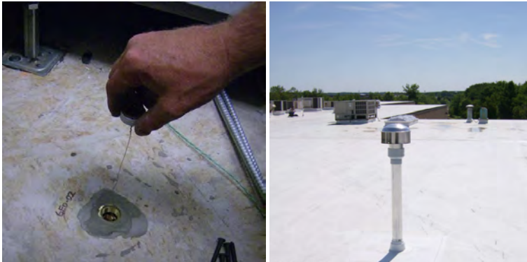
Geosyntec initiated a vapor intrusion sampling (left) and passive mitigation (right) program that reduced our client's long-term liabilities by almost 90%.
