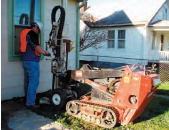
Soil gas probes were installed adjacent to residences as part of the TriHydro program to assess the presence of vapors.
