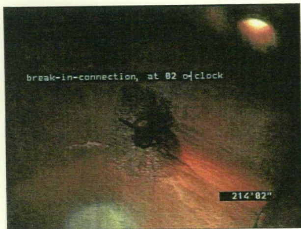
IMAGE: 6a, TAPE #: 01, 00:00:00 214.2FT, break-in-connection, at 02 o'clock
