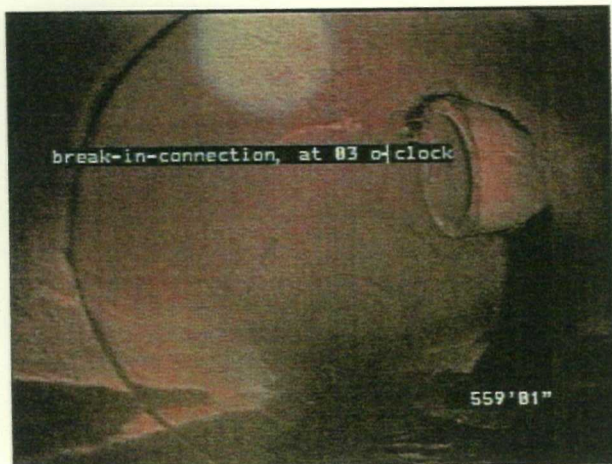
IMAGE: 15a, TAPE #: 01, 00:00:00 559.1FT, break-in-connection, at 03 o'clock
