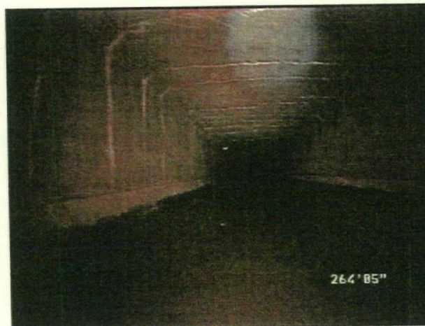
IMAGE: 7a, TAPE #: 01, 00:00:00 264.4FT, Multiple Cracks, from 08 to 04 o'clock
