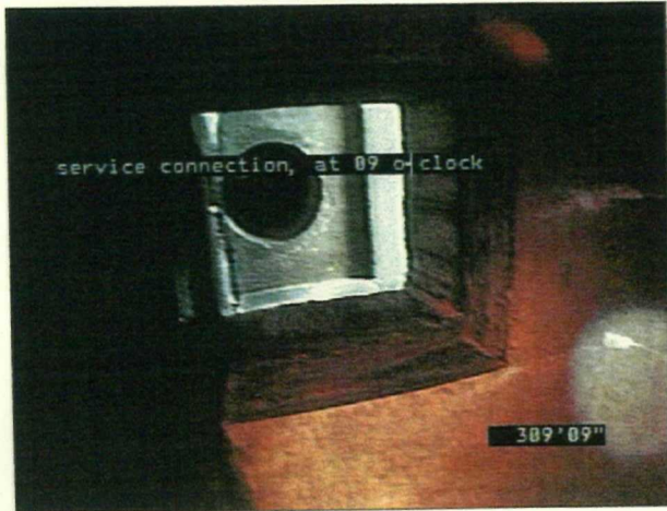
IMAGE: 8a, TAPE #: 01, 00:00:00 309.75FT, service connection, at 09 o'clock
