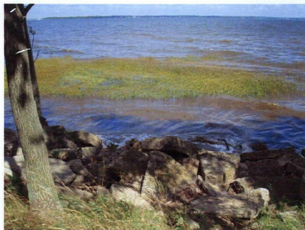
Figure 5: Seawall Slag at High Tide
