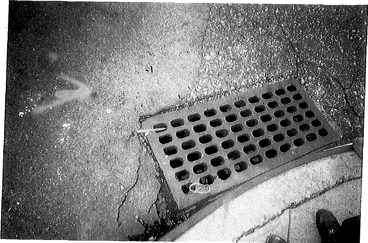
Photo 1 Storm drain located at the intersection of Bond and President Streets. 1130
