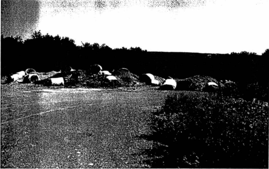
July 31, 2007: Bales of hay holding down plastic tarps which cover some of the piles of construction debris.
