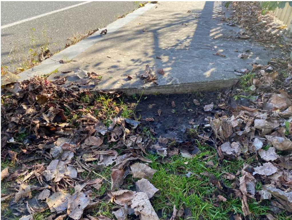
Photo 6: Approach sidewalk settlement at the west end of the south sidewalk.
