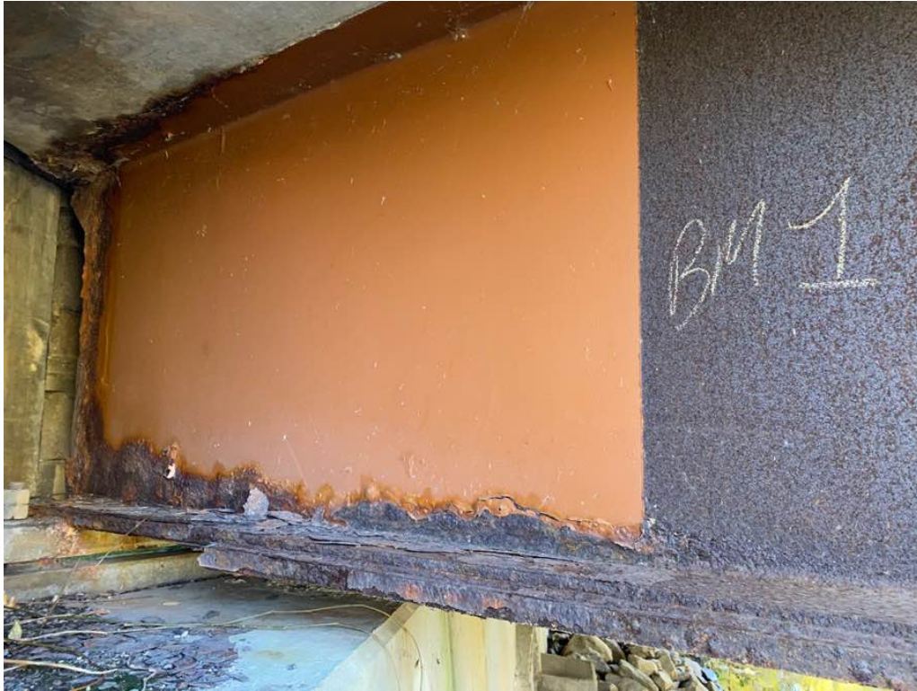
Photo 7: Rusting with delamination at the east end of beam 1. Also, note the delamination in the cover plate and the associated welds.
