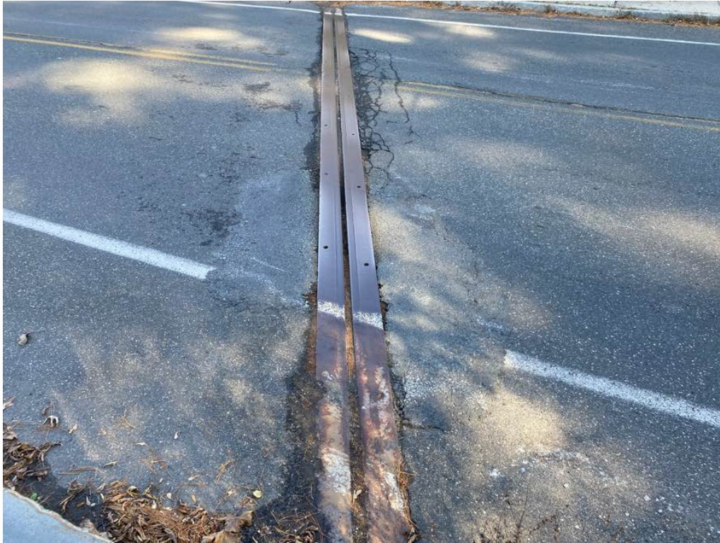
Photo 3: East deck joint filled with sand and debris. Note the approach pavement pulling away from the armor and patches.
