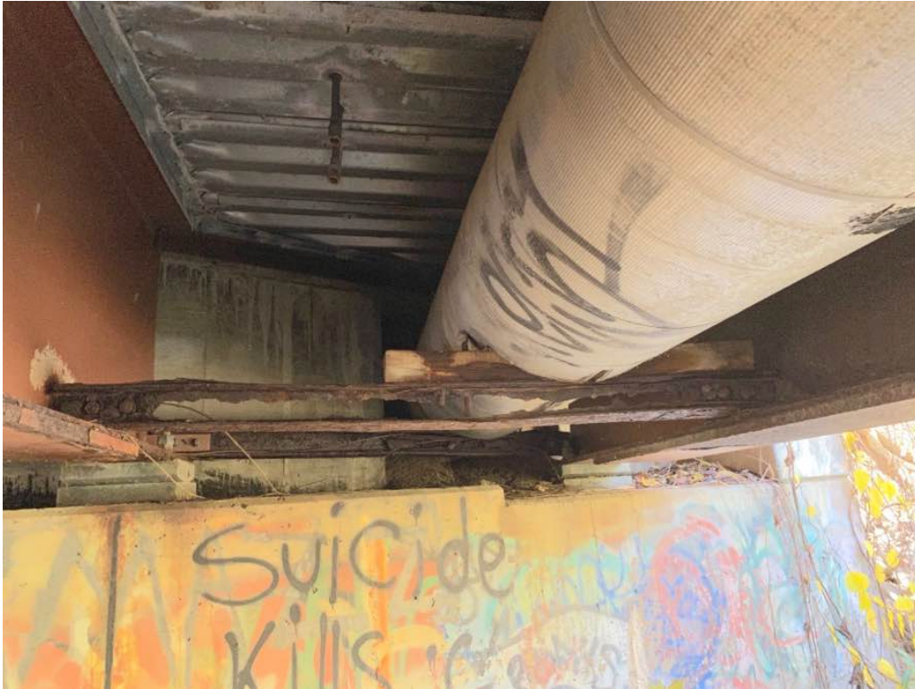
Photo 5: Rusted utility support at the west end of bay 1. Also, note the fill spilling through the utility bay in the backwall.
