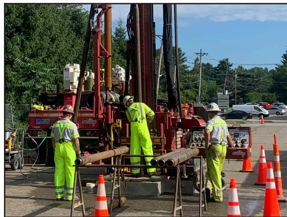
Workers drilling a new monitoring well as part of the ongoing groundwater investigations.
