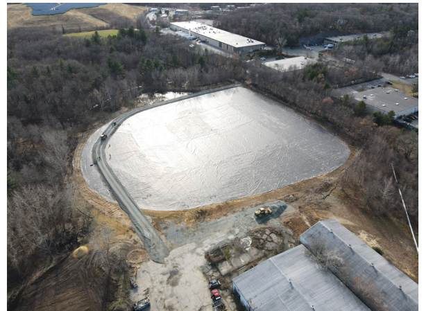
Aerial image of the Containment Area feature (engineered slurry wall and temporary cap) on the Olin property. Olin Corporation replaced the previous cover of the Containment Area in the fall of 2021.
