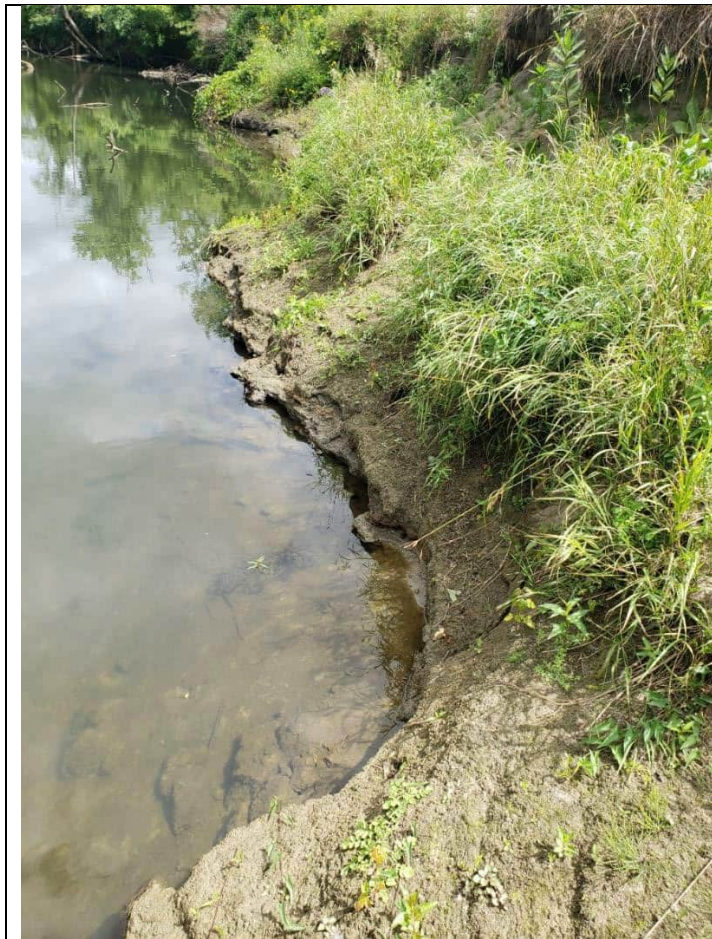
Left bank near Station 233; bank swallow cavities
