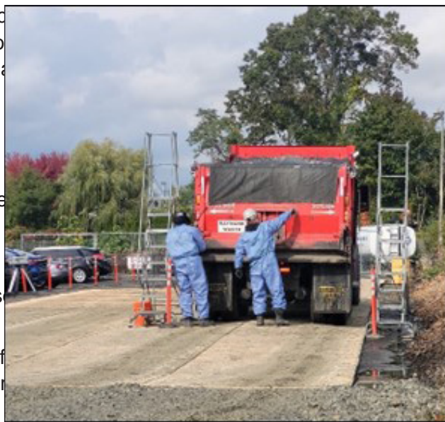
Example of secured truck used at the Raymark Superfund Site in Stratford, Connecticut
