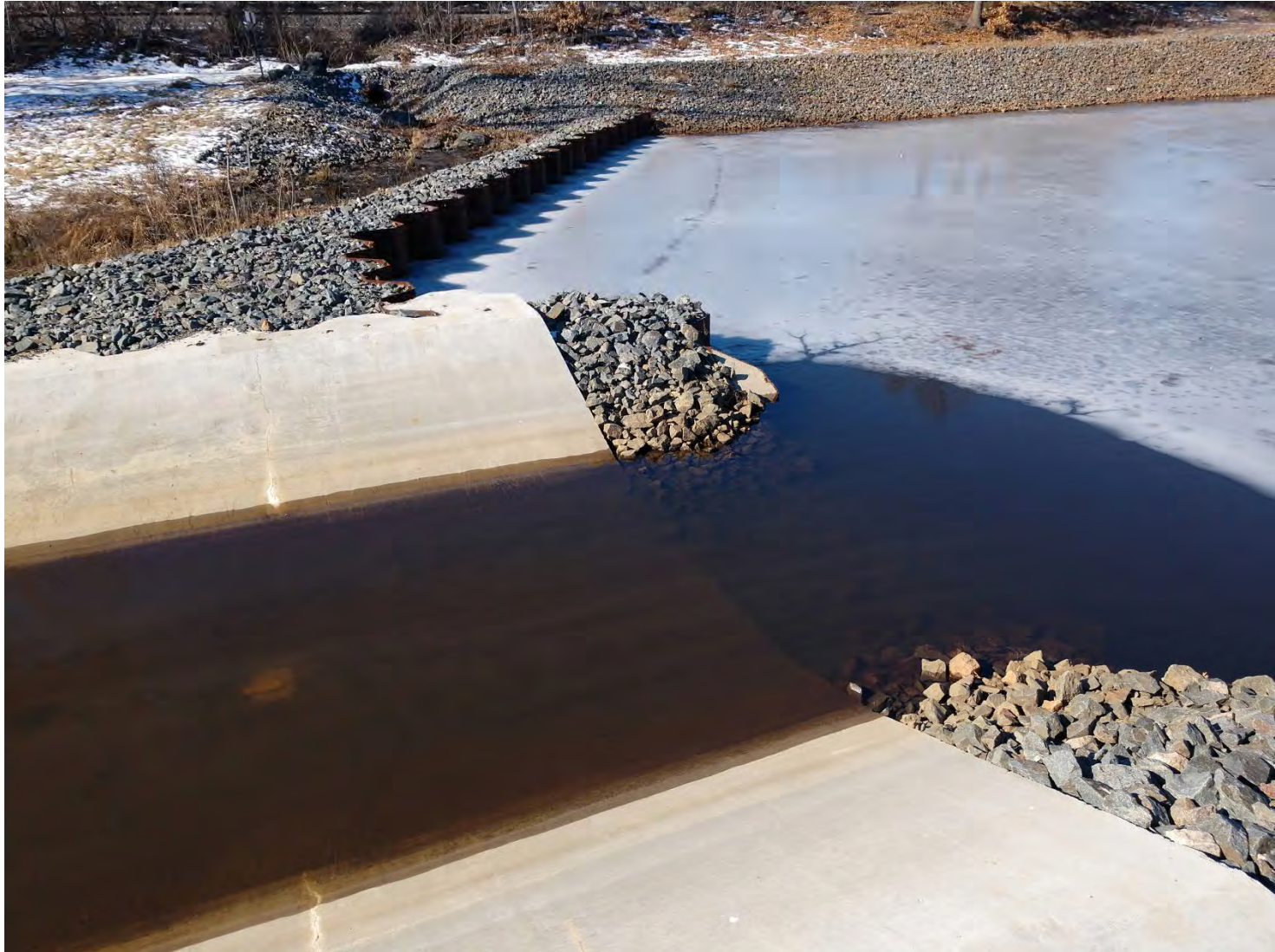
Halls Brook Holding Area Pond Outlet Structure
