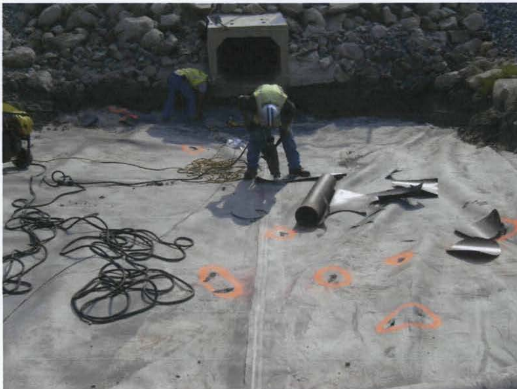
6) Repair of liner damaged during removal of VSL soil layer. 8/25/08
