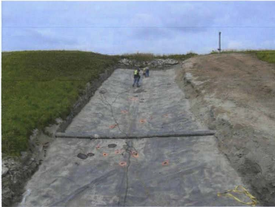
7) Repair of liner damaged during removal of VSL soil layer. 8/25/08
