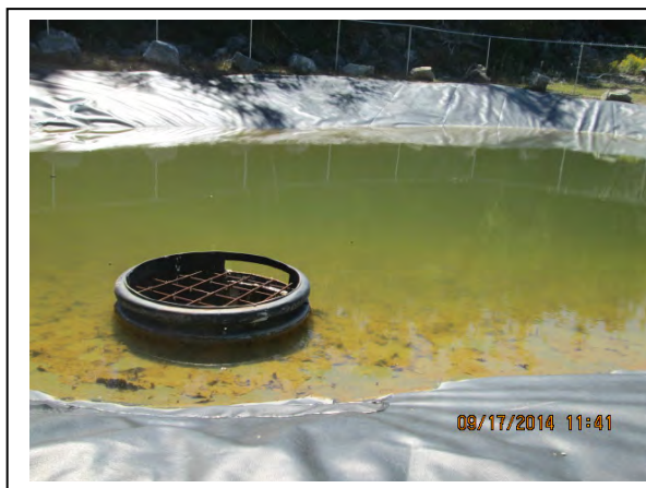
Stormwater pond outlet structure at Mine Ops Area
