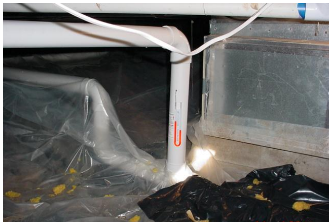
Figure 4-4. Crawl-space mitigation using submembrane depressurization. Courtesy Kansas Department of Health and Environment
