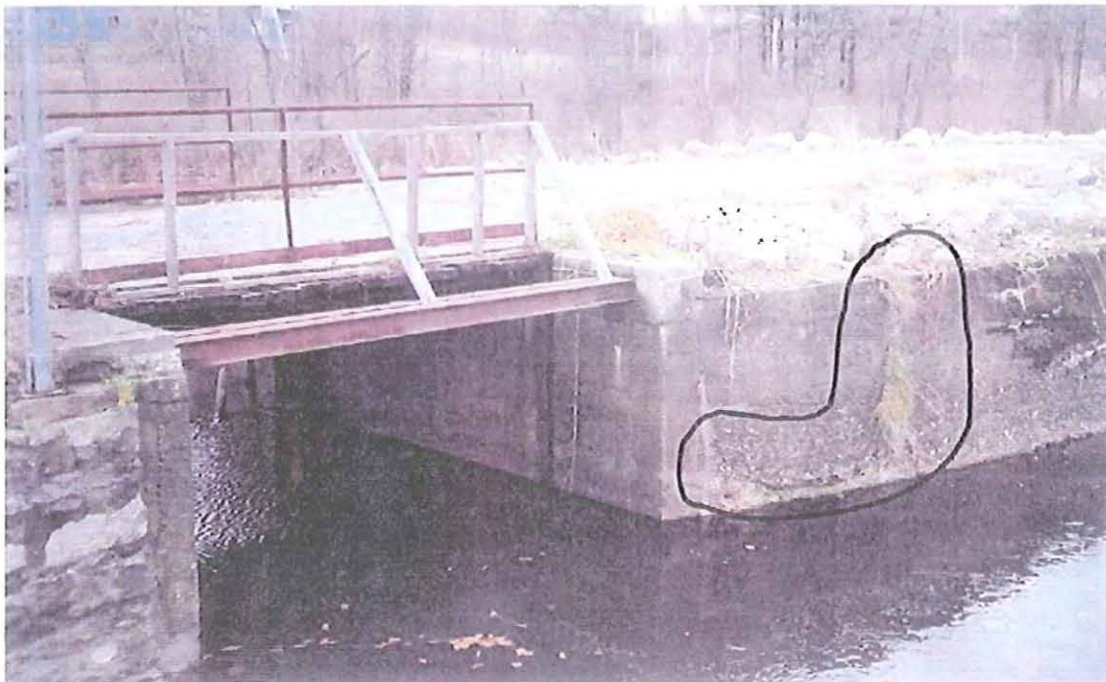
Photo 14 Upstream face of raceway stoplog sluice structure. Note damage at waterline and vertical crack (with vegetation) on right wall.
