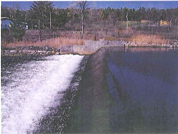
Woods Pond Dam Quarterly Inspection – April 27, 2006 Crest of Spillway Looking East to West
