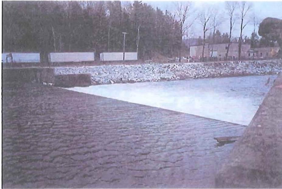
Photo 1 View of reservoir, overflow spillway and left walls and abutment from upstream of right abutment training wall.
