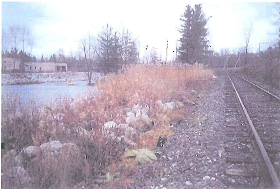
Photo 3 Riprap protection along right bank upstream of overflow spillway; railroad at right abutment. Viewed from the right bank upstream of the overflow spillway.
