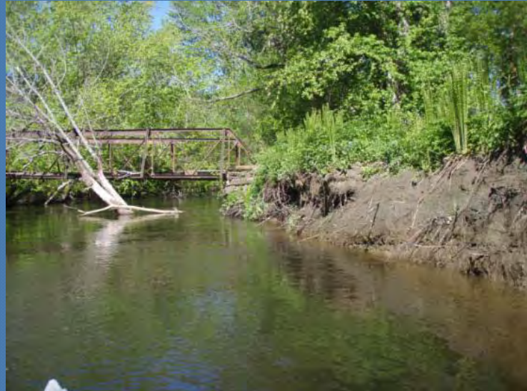
Bank Erosion Floodplain Deposition
