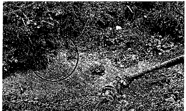
Water distribution pipe laid in drainage ditch. Note home sewage outfall circled in picture, not uncommon in rural areas.
