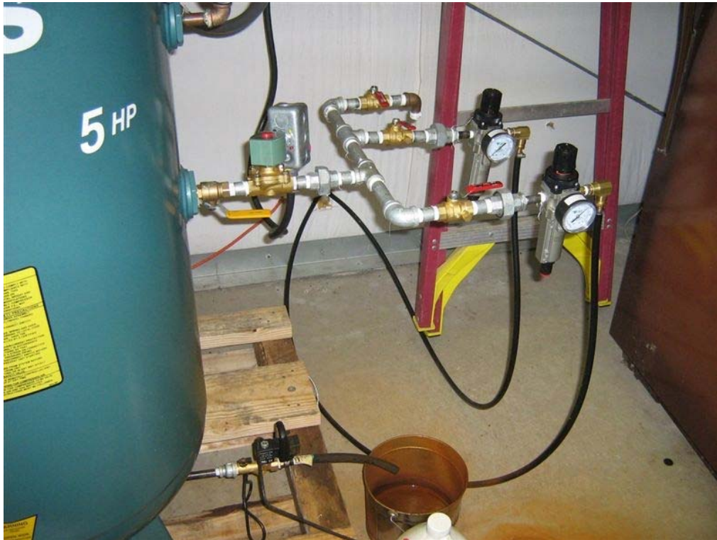
3. Air line manifold, air filter/regulators, and compressor auto drain.
