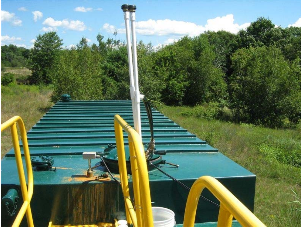
5. Siphon relief valves located at top of fractionation tank.
