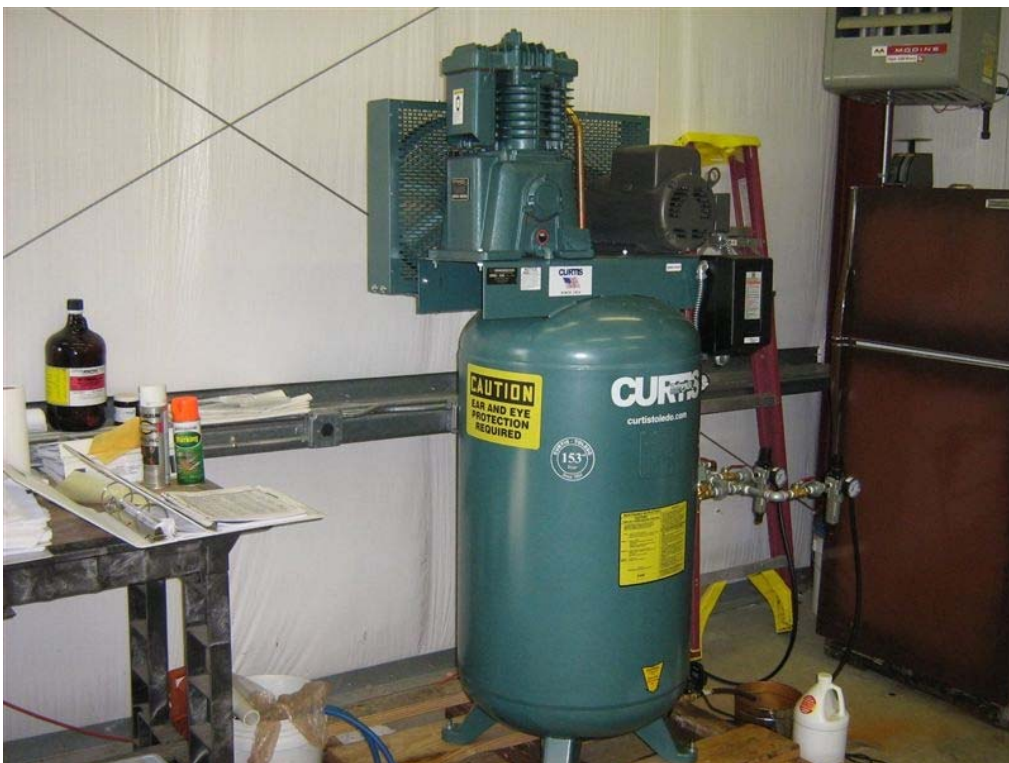
2. 80-gallon reciprocating air compressor inside Butler Building.
