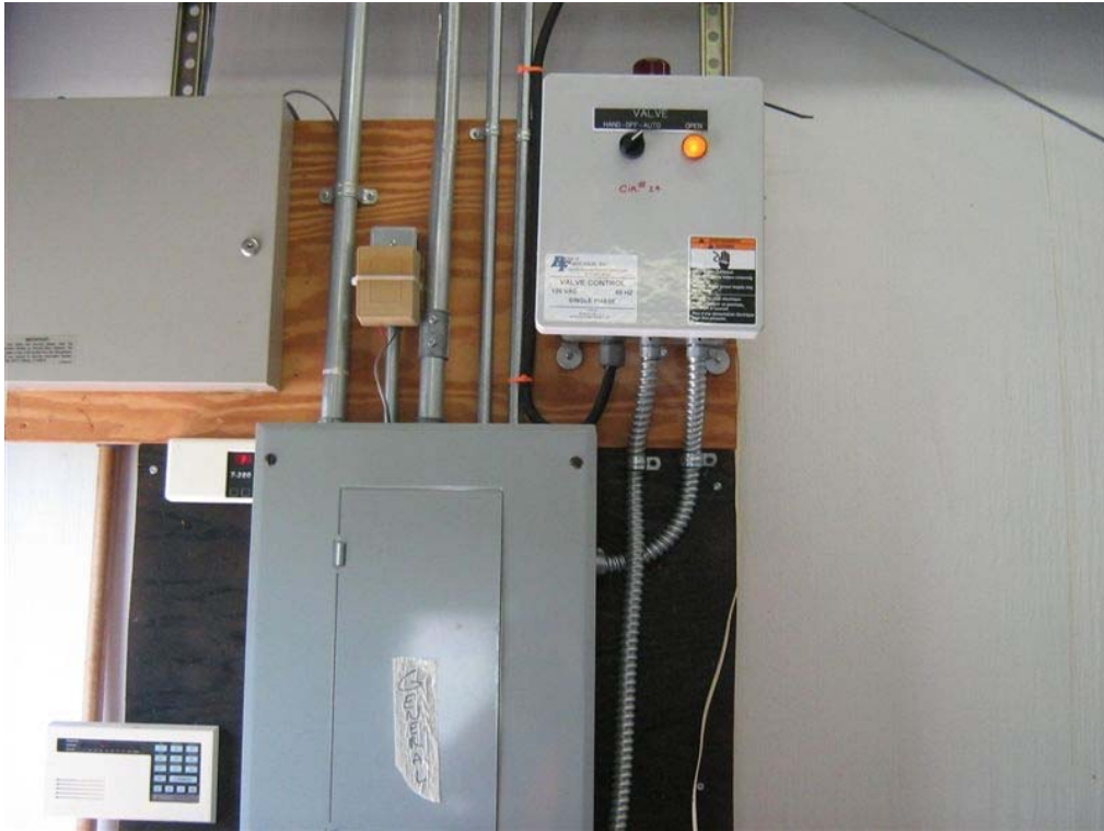
1. GWE system control panel (top right), main electrical control panel (bottom center).
