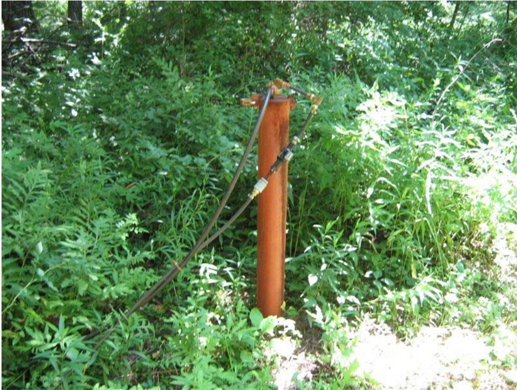
7. Pumping well SB-4D.
