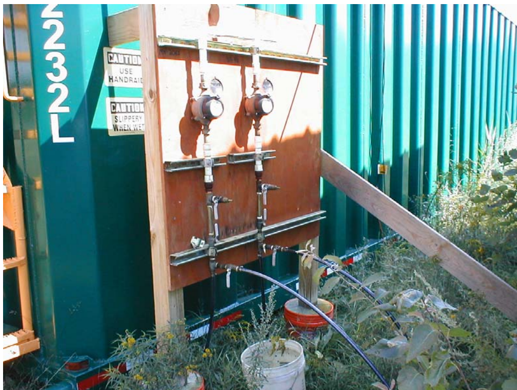
4. View of manifold, including; totalizers, influent sample ports, and manual flow ports.
