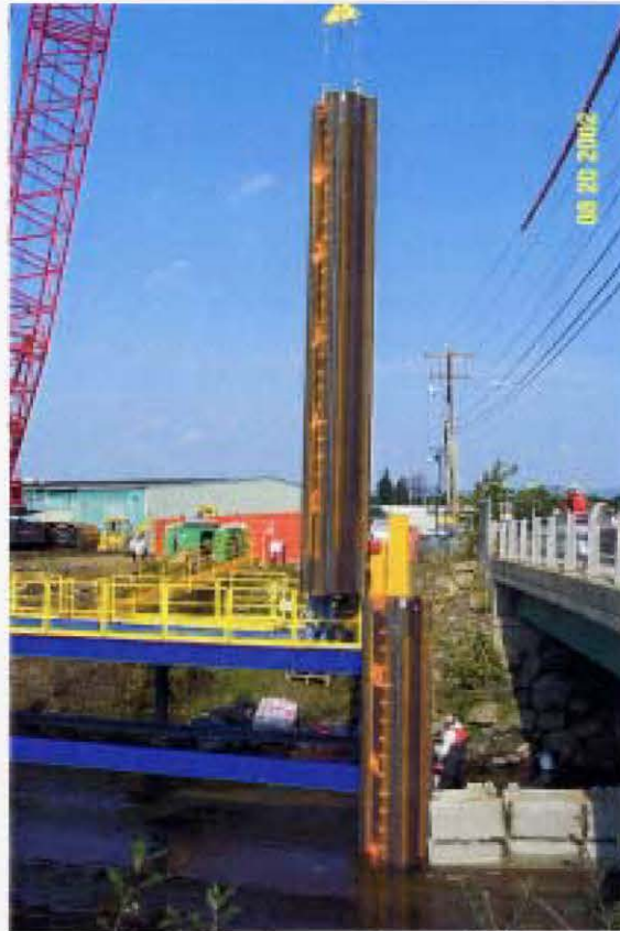
Photograph 3 – Installation of Sheet Pile Wall Immediately Downstream of the Lyman Street Bridge
