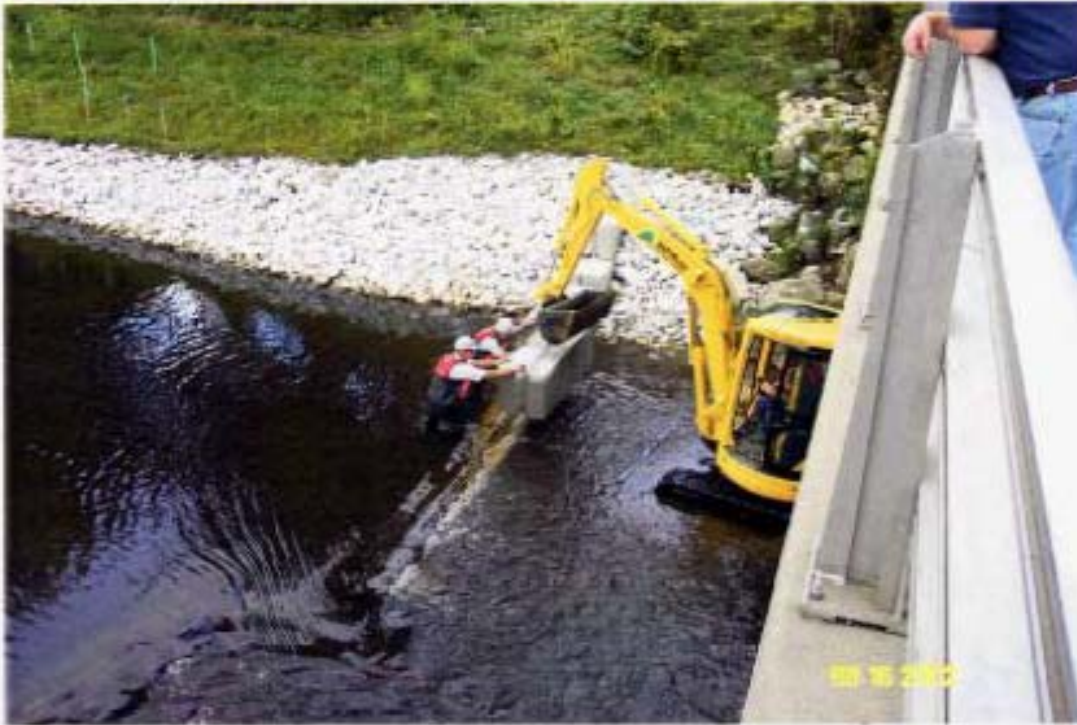
Photograph 1 – Placement of Bin Blocks Upstream of Lyman Street as Part of Remediation Cell No. 1A
