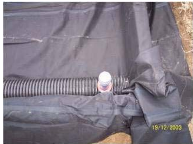
Figure 6-3. Internal Water Reservoir System
