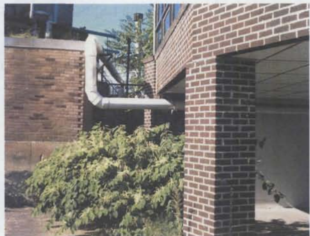
Vapor line along Matheis Court Building
