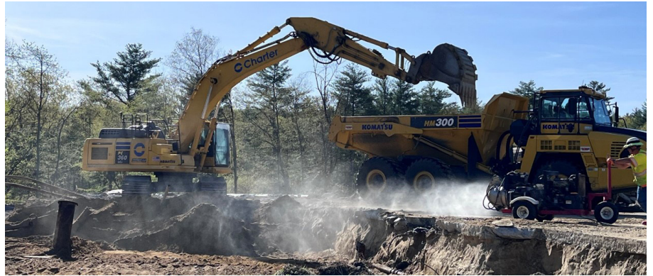
Photo 2: Mister spraying water over Building D soils and excavation area. The wetting of the soil and work area minimizes dust generation.
