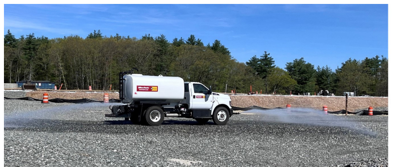
Photo 6: The site roadways are wetted multiple times per day with a water truck to decrease dust generation due to on-site truck traffic.
