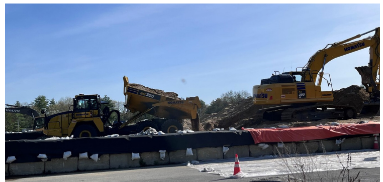
Photo 4: Excavated soils are transported via off-road dump truck to the on-site Waste Processing Area (WPA).
