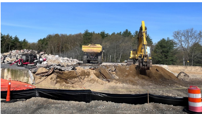
Photo 3: Soil excavation from Building D area. Soils are loaded into an off-road dump truck for transport to the on-site site Waste Processing Area.
