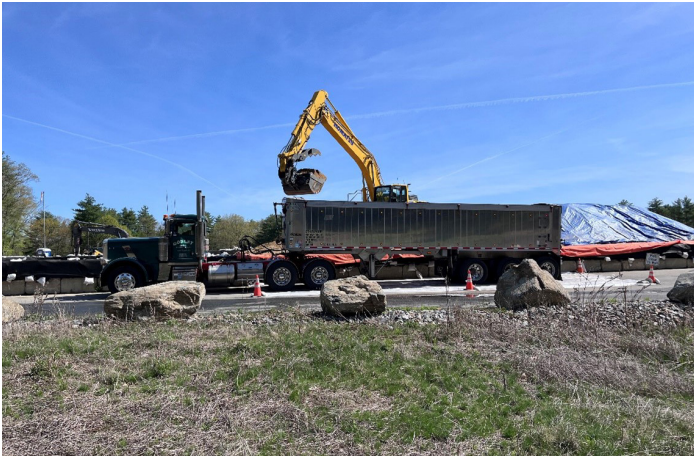
Photo 7: Lined, dump trailers are filled with soil. Each truck is lined and covered prior to leaving the Site. Between 30-35 tons of soil are put into each truck.
