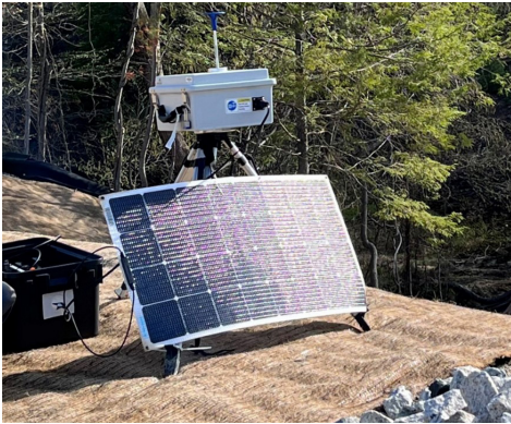
Photo 1: Dust monitoring stations are installed around the perimeter of the work area to monitor ambient dust levels during work. The dust monitoring stations record dust levels in real time and are monitored by project personnel.
