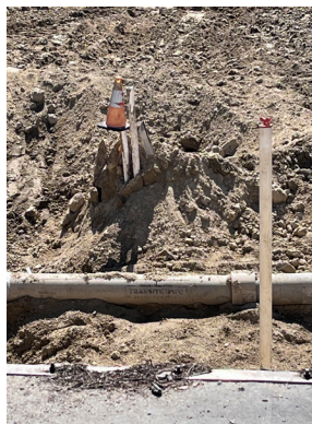
Asbestos transite pipe uncovered at Site
