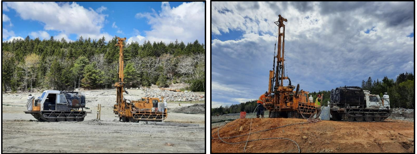
Photo 6. Views of geotechnical and well abandonment on top of the Tailings Impoundment with New England Boring Contractors.
