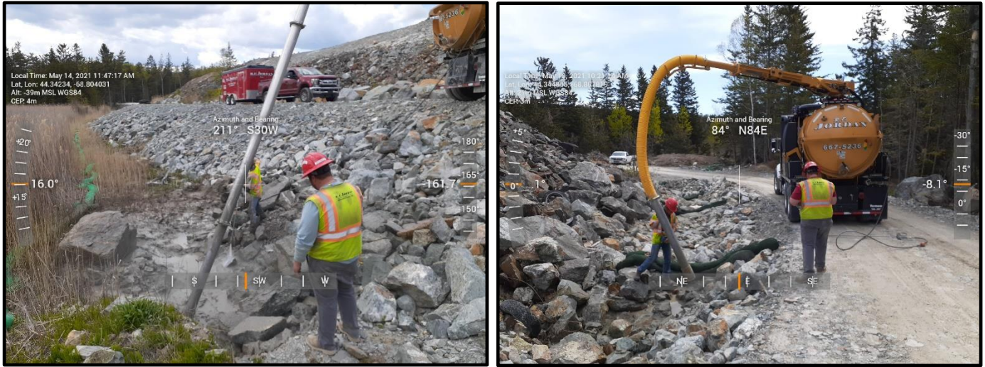
Photo 2 (group). Views of RF Jordan removing tailings sediment from toe of the East access road and along access road drainage features.
