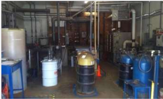
Photo 5. Pump and Treat System.
