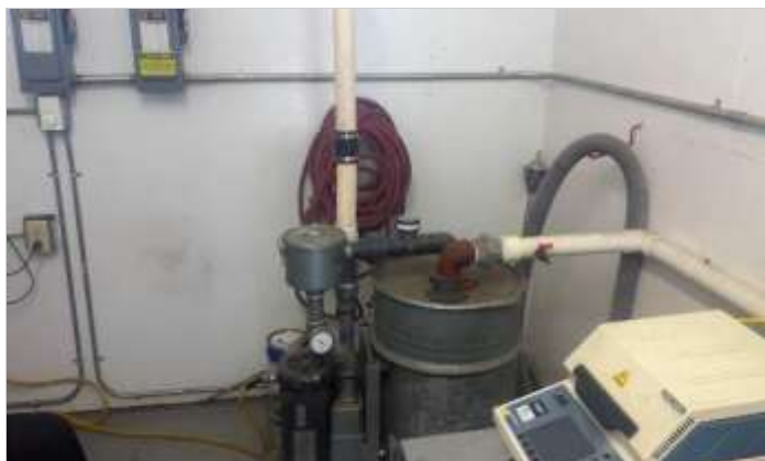
Photo 1. Soil Vault SVE System
