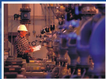
FS-12 Treatment Facility
