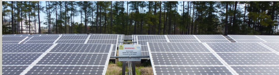
Solar panels on the capped part of the site.
