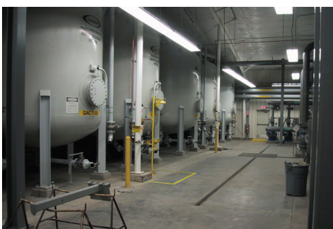
Indoor treatment facility
