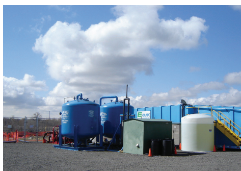
Outdoor treatment facility
