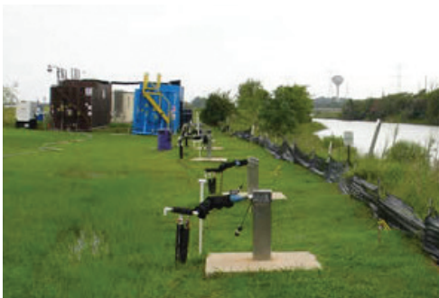
Groundwater pumping wells
