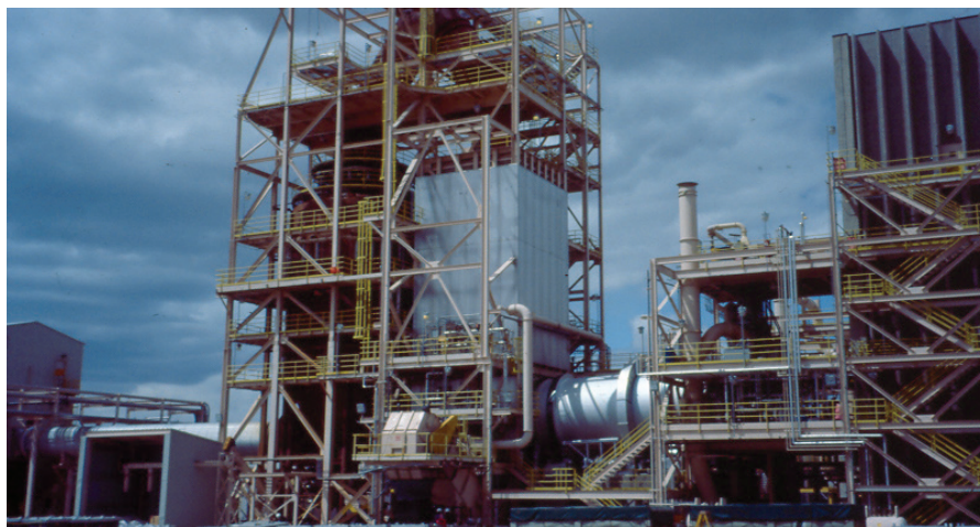
Example of an offsite incinerator.
